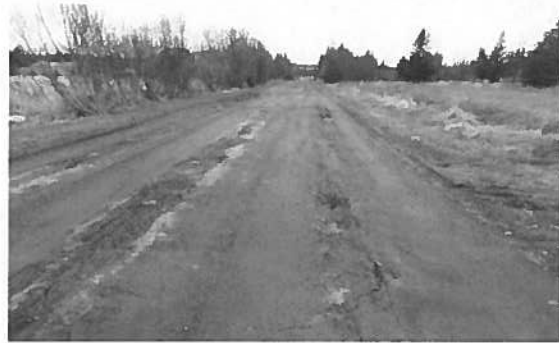
Eagle Pl: Gravel road with subsidence issues, and inadequate drainage
