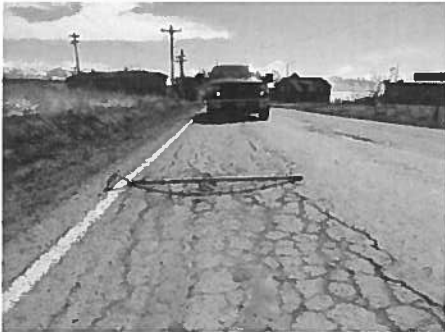
Ohlsen Ln: Paved road with multiple issues including major cracking, subsidence, and out of spec road corridor
