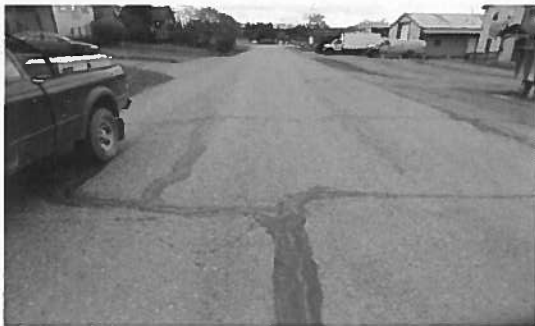
Extensive crack repair on Grubstake Ave. (West) Crack sealing is an annual maintenance task
