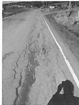
Cracking and pothole formation on Ohlsen Ln. Narrow road corridor causes out of spec travel lanes, shoulders and
