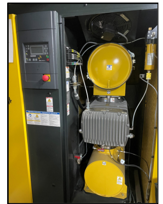
Control panel and inside mechanisms
