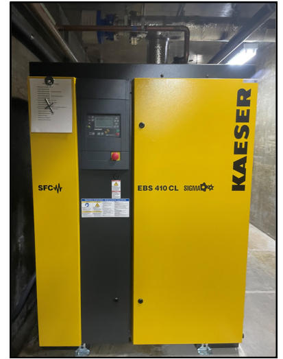
New Kaeser blower unit
