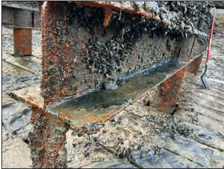
Figure 1-5. Heavy Corrosion in Primary Structural Beams
