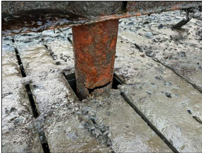
Figure 1-10. Hole in Pile Under Beam 7
