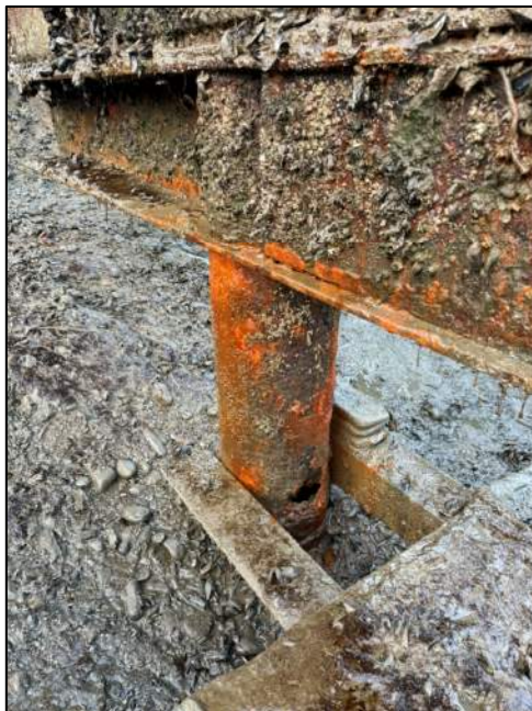
Figure 1-11. Hole in Pile Under Beam 5
