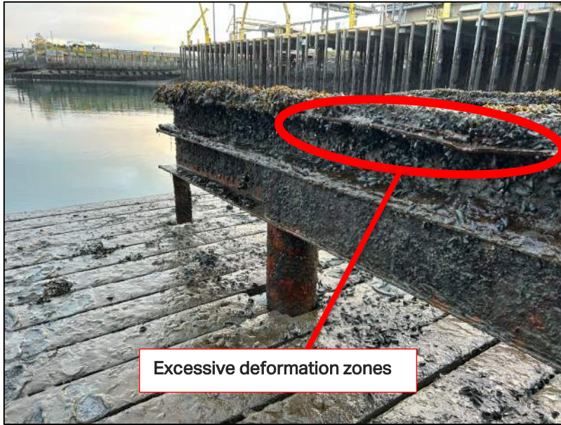
Figure 1-7. Excessive Deformation in Beam Flanges
