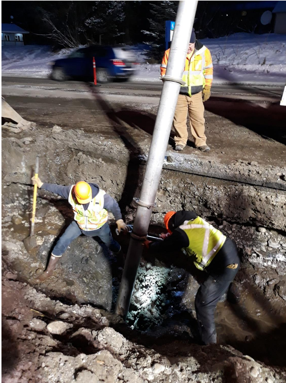
The photo above shows Paul Raymond (at street level), Jason Hanenberger, and Mike Szocinski working on the Pioneer Avenue water main break.
