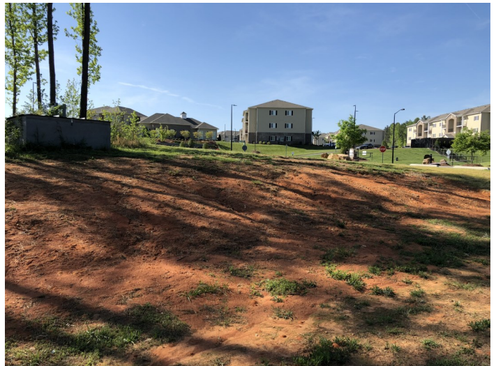
Eroding slope beside multi-use field
