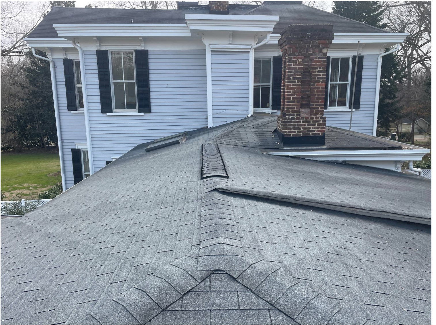
Current photo of multiple rooflines looking south from roof of brick furnace building
