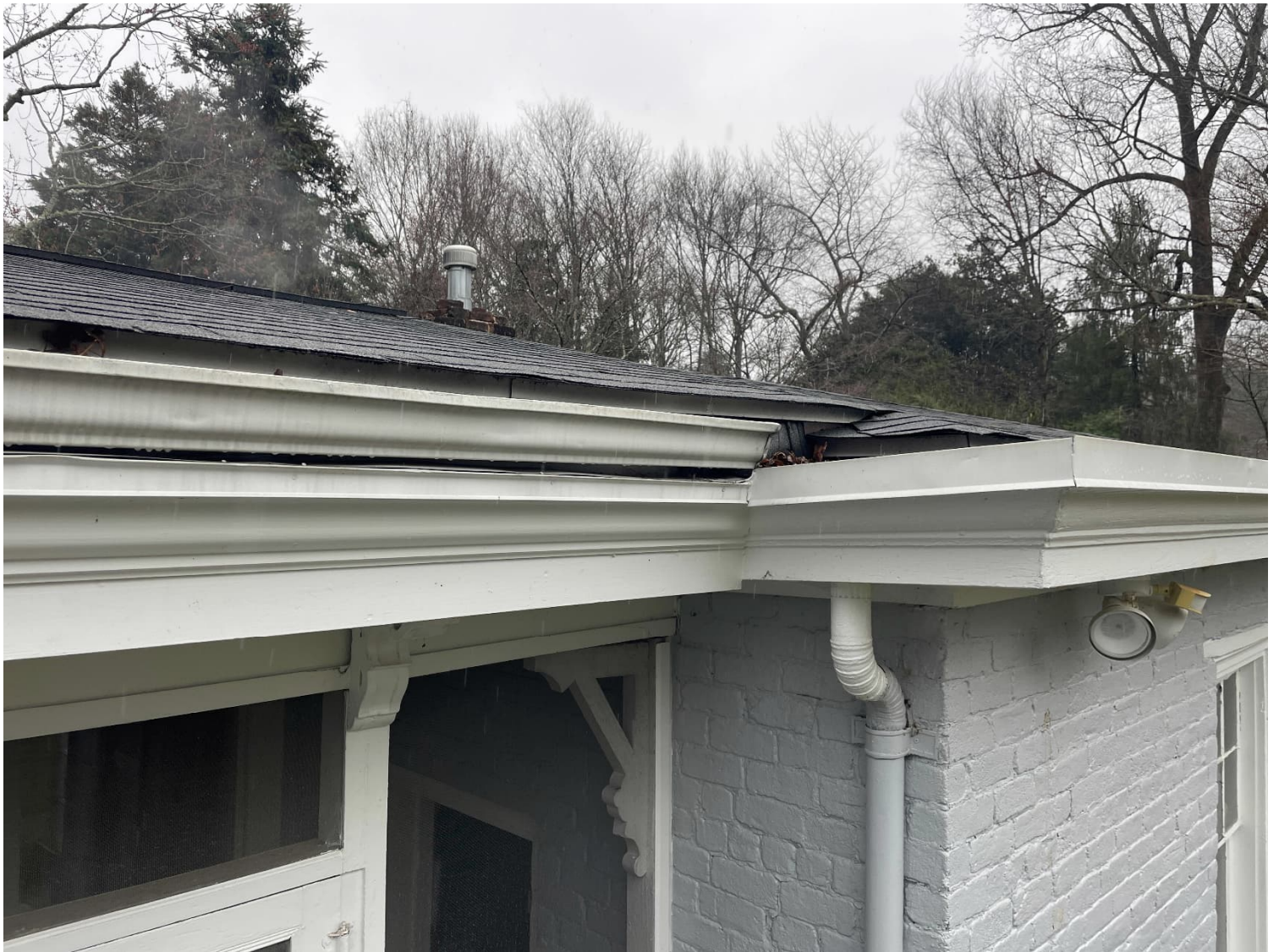
Current photo of awkward intersection of roof/double fascia into brick furnace building roof
