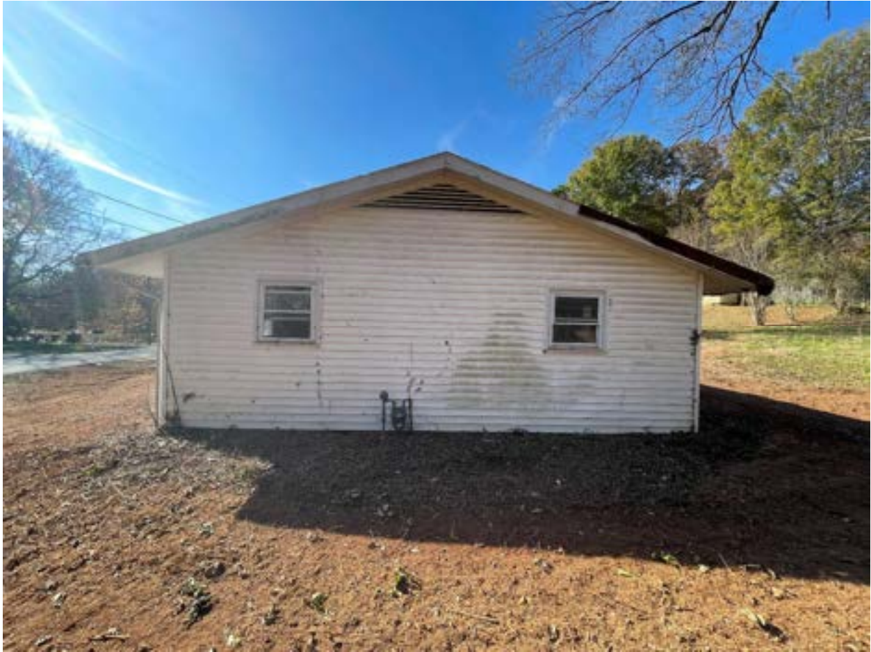
Right Side/East– proposed replacing vinyl windows with wood windows, new rear addition with asphalt shingles and brick foundation to match, wood windows, Hardie siding, Miratec trim and wood deck
