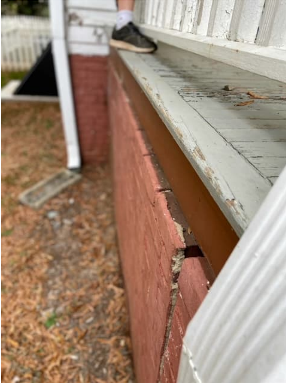
Photo showing failing curtain wall
