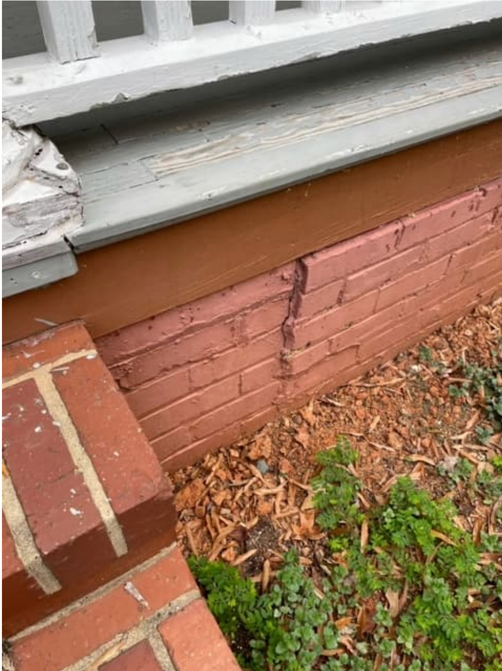
Photo showing failing curtain wall
