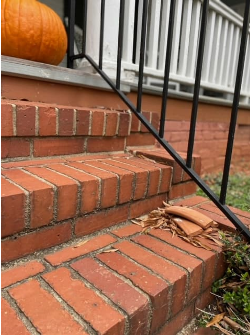
Photo showing failing front steps
