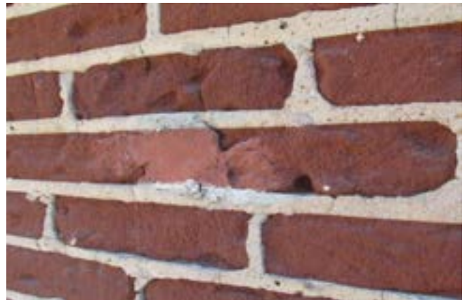
Sandblasting brick permanently damages masonry surfaces.
