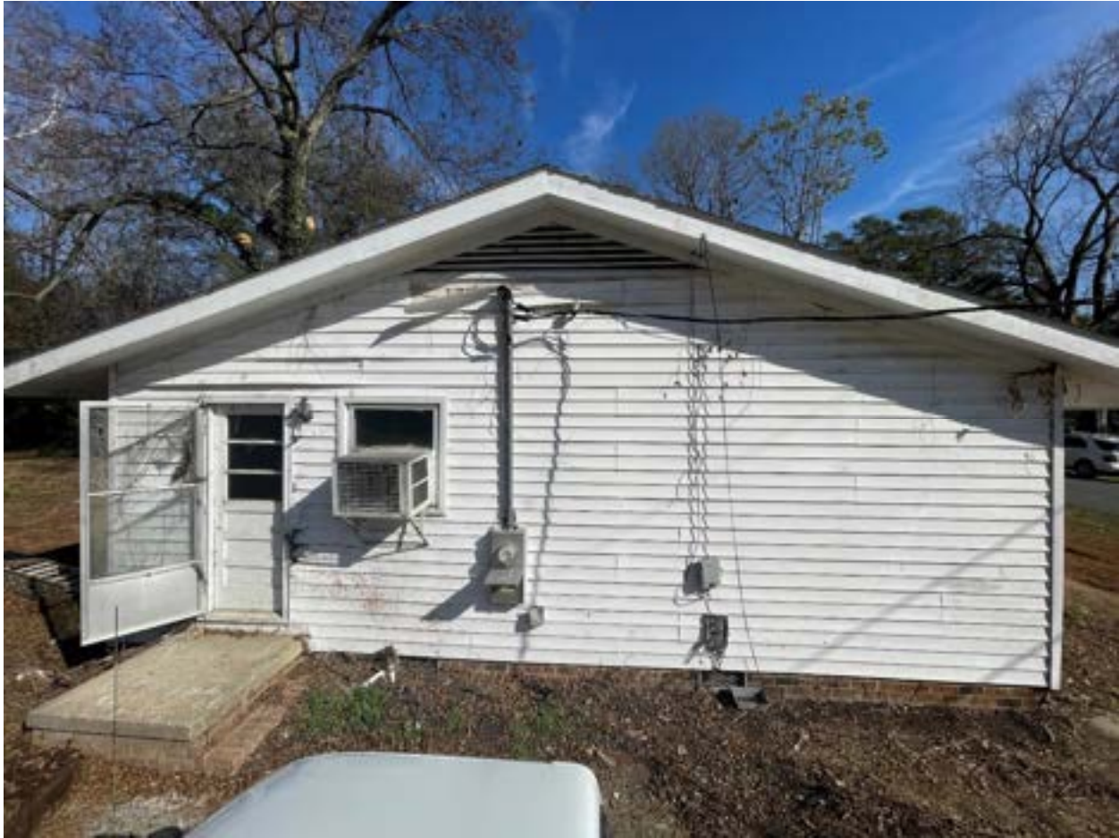
Left Side/West- existing stoop and door to be removed, proposed rear addition with asphalt shingles and brick foundation to match, wood windows, Hardie siding, Miratec trim and wood decks
