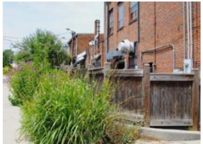
HVAC units and trash containers are screened from view through the use of fencing and plantings at this commercial building at 101 N. Churton St.
