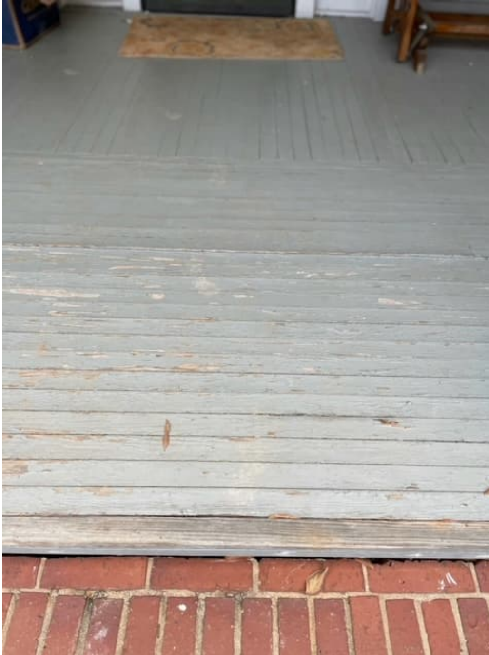
Photo showing incorrect repair of porch flooring
