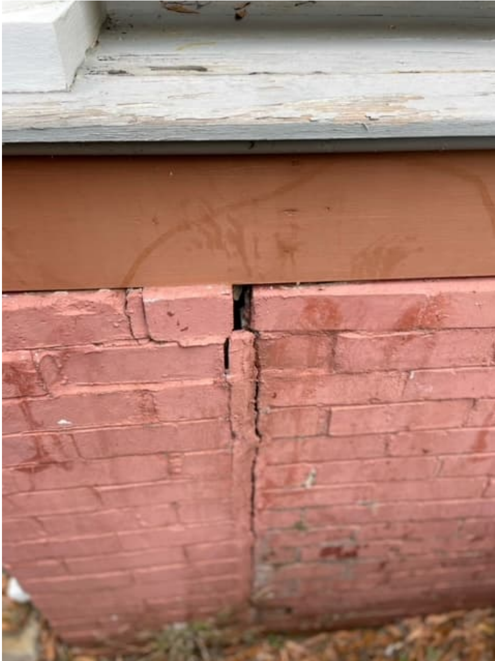
Photo showing failing curtain wall and failing pier
