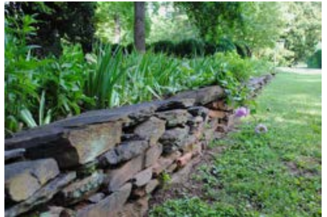
This retaining wall at 131 E. Queen St. is constructed from stone from the Duke quarry and is typical of retaining walls found throughout the historic district.
