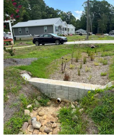
The Award-Winning Odie Street Stormwater Green Infrastructure Project
