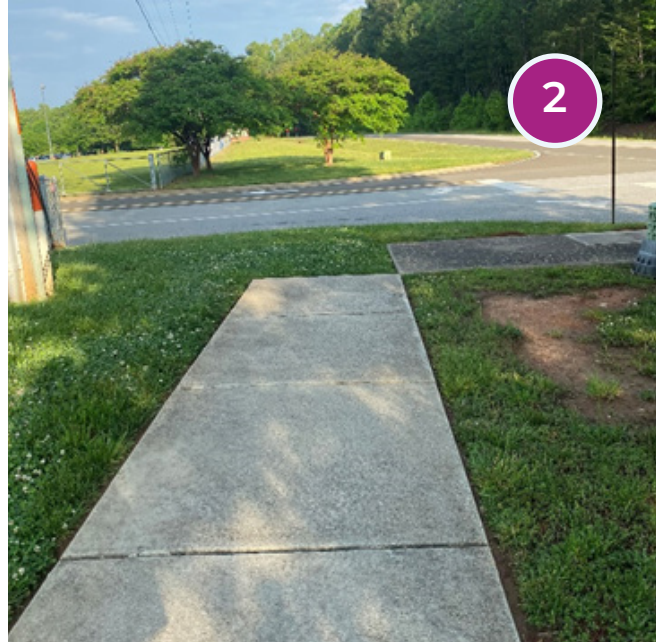
End of sidewalk at the eastern driveway
