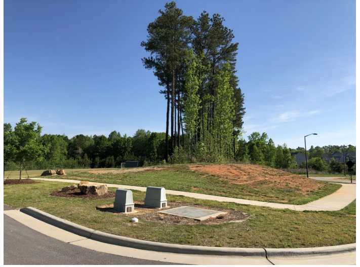
Eroding slope at entrance to Cates Creek Park
