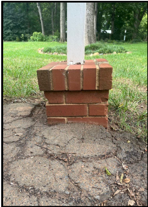
Brick support pier without footings (4 total)
