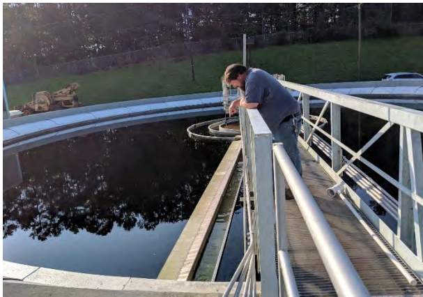
A utility mechanic inspects a mechanical arm on the Wastewater Treatment Plant's clarification tank, which sweeps the water surface of large organics and trash.
