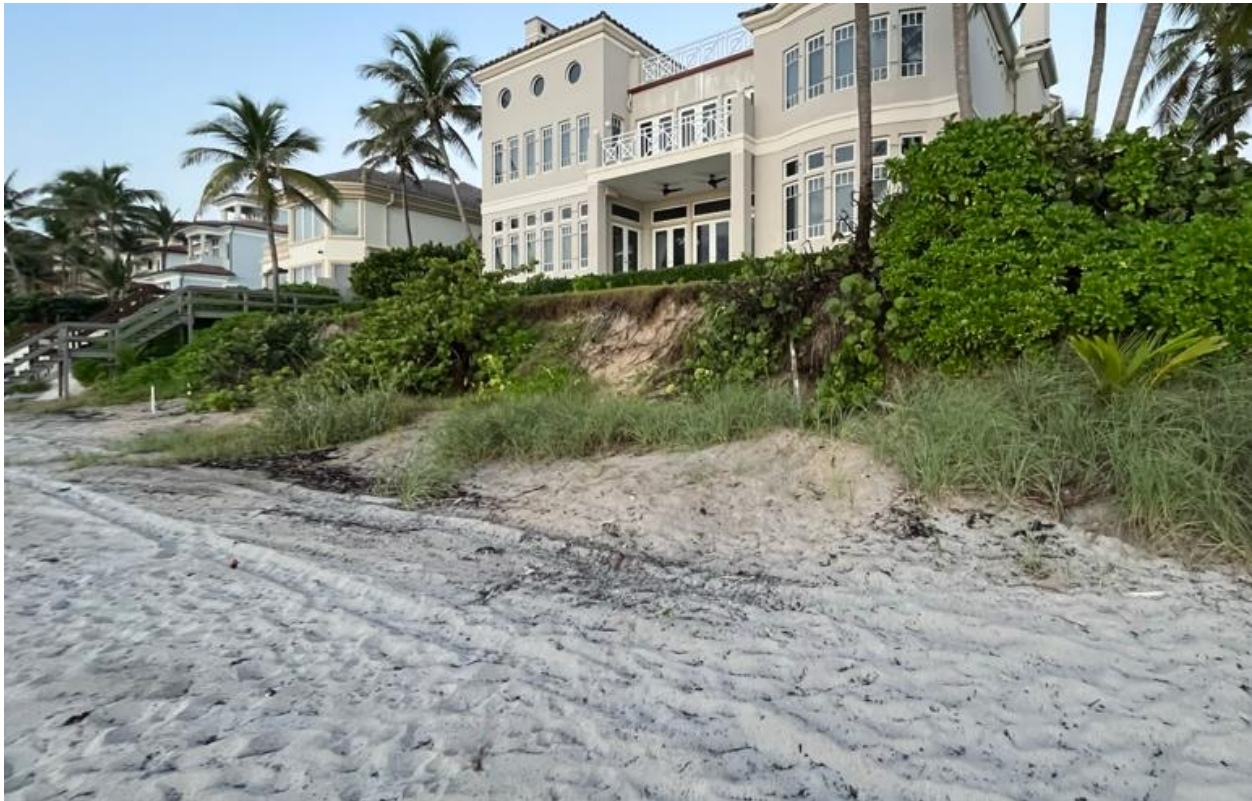
Photo 11. The most significant erosion observed in the Ocean Place Estates.
