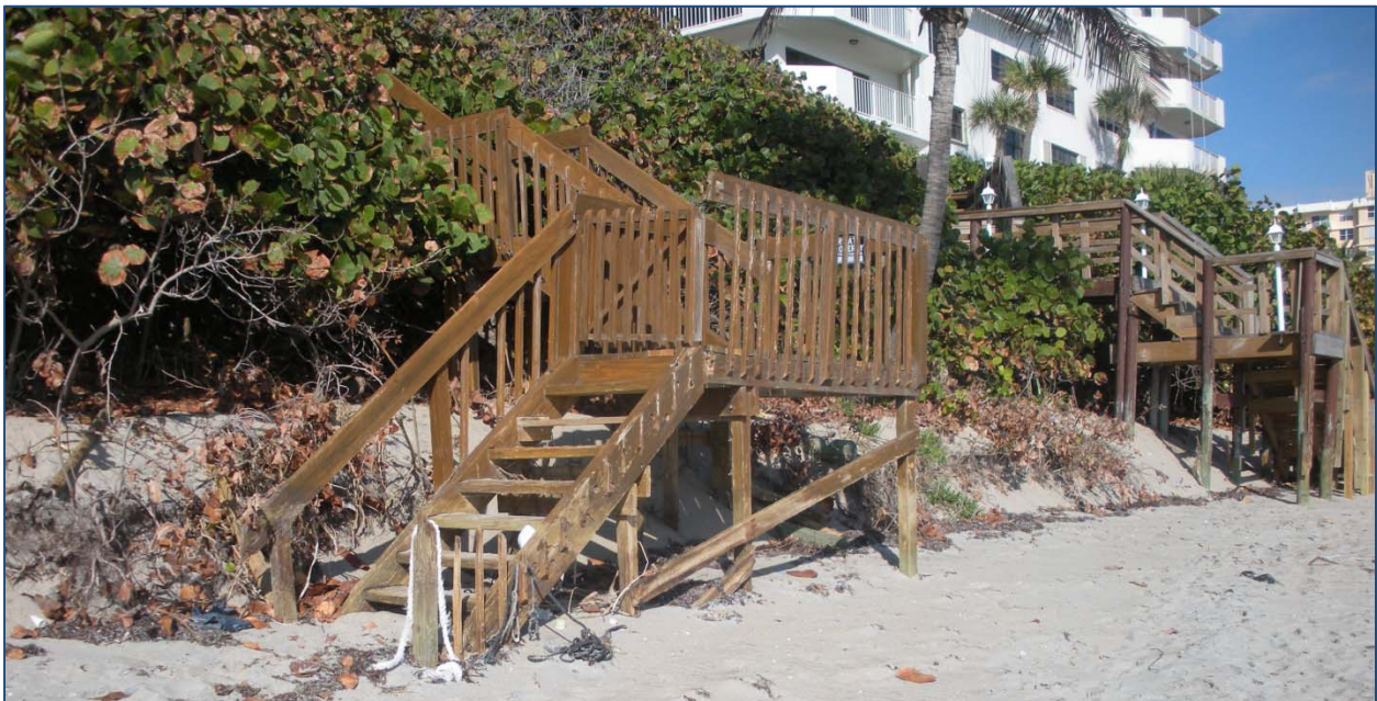
Photo 7. View of a scarped dune and beach erosion. Note that there is an approximate paint line on the staircase, which generally indicates a previous beach elevation and shows erosion of the beach. The missing handrail suggests recent damage from Hurricane Sandy.
