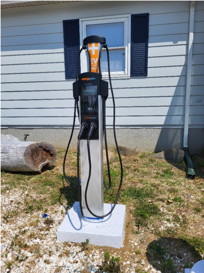
Photo 2: Existing EV infrastructure
