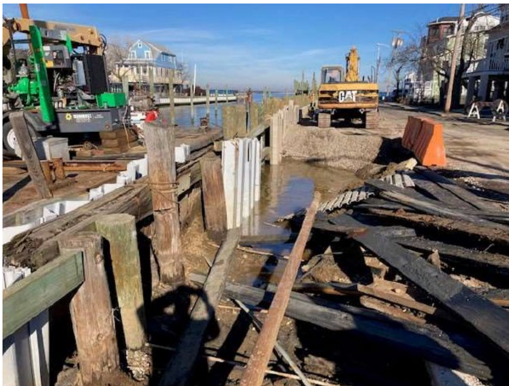
Erosion right up to roadway
