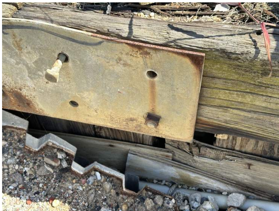
Photo 18: Section B , Southernly Bulkhead, Fastener & Metal Sheetpile Bulkhead Condition, View 2
