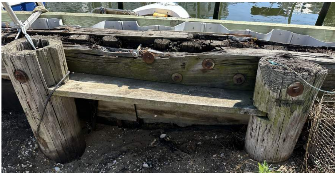
Photo 27: Section C , Westerly Bulkhead, Deteriorated Timber Elements & Fasteners, View 2
