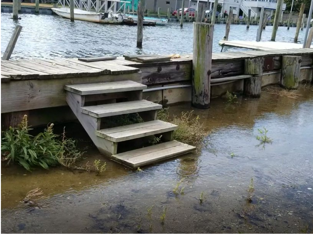
Flooding observed along the Captain's Cove bulkhead (9-30-2019) (Provided by William Brunt)
