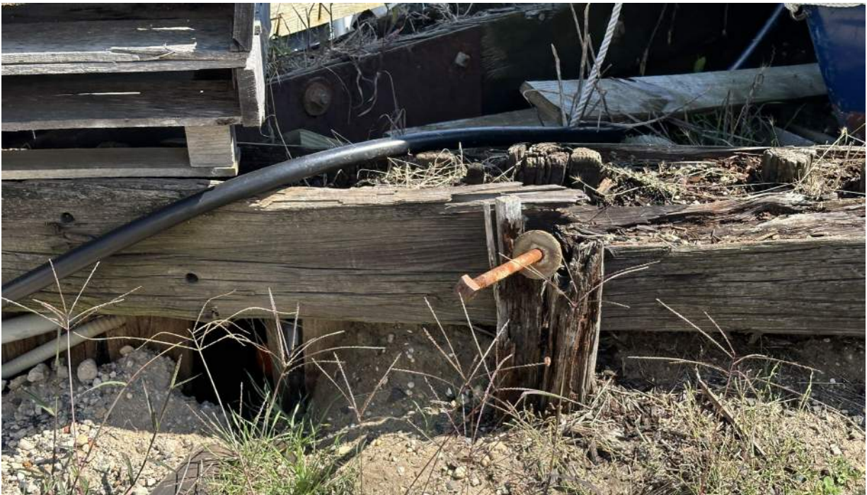
Photo 17: Section B , Southernly Bulkhead, Fastener & Metal Sheetpile Bulkhead Condition, View 1
