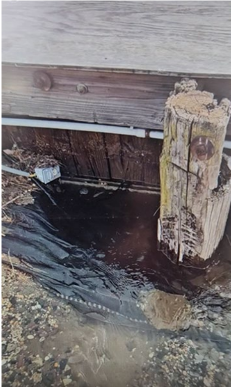
Flooding observed at the bulkhead (February 2024) (Provided by William Brunt)
