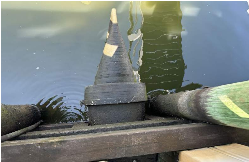
Photo 11: Section A , Easternly Bulkhead, Outfall Pipe with Outfall Backflow Preventer (Tideflex)
