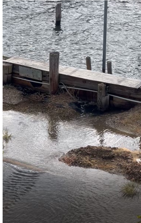
Flooding observed at the bulkhead (September 2024) (Provided by William Brunt)
