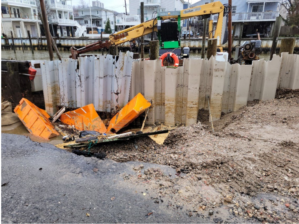
Photo depicting poor condition of the bulkhead along Washington Avenue (December 2022) (Provided by Michael Muscillo)
