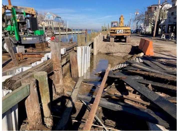
Erosion right up to roadway
