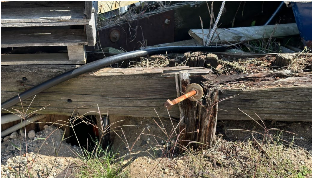
Southernly Bulkhead, Fastener and metal sheetpile bulkhead condition (From Colliers Engineering and Design's Report dated November 4, 2024)
