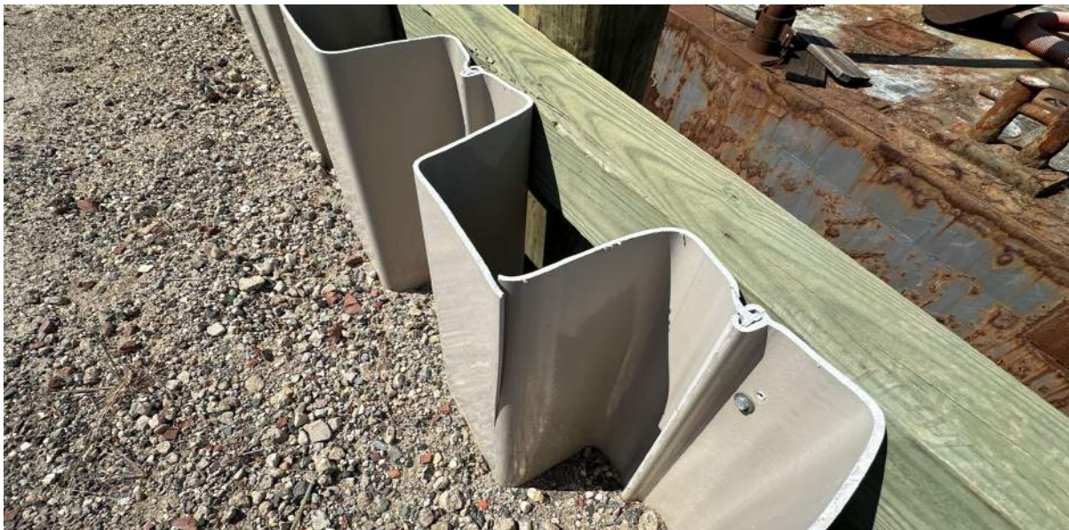
Photo 9: Section A, Easternly Bulkhead, Cracked Sheet Pile Section
