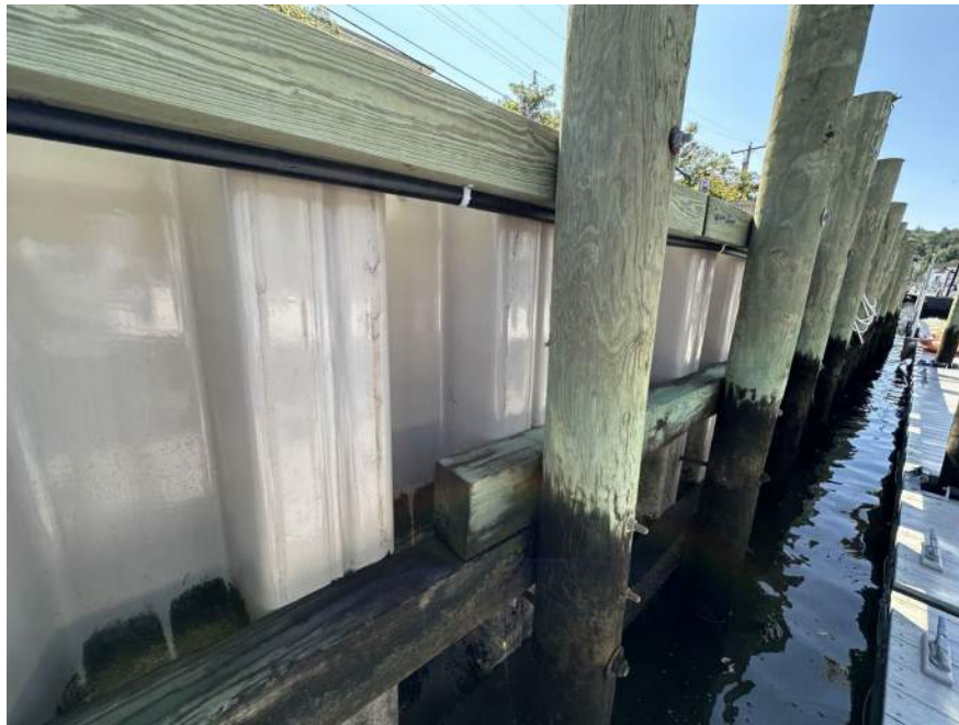
Photo 3: Section A, Eastern Bulkhead Piles, Sheet Piles and Walers Viewed from Floating Dock Infront of Bulkhead
