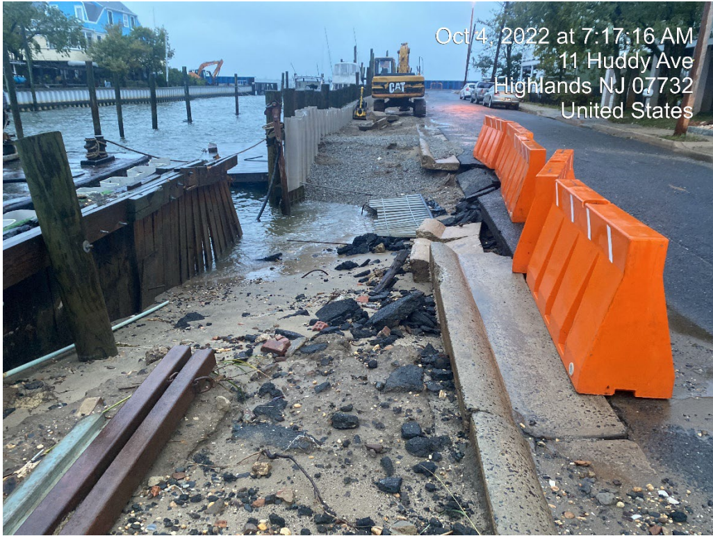
Damage to the Washington Avenue Right-of-Way (10-4-2022)(Provided by William Brunt)
