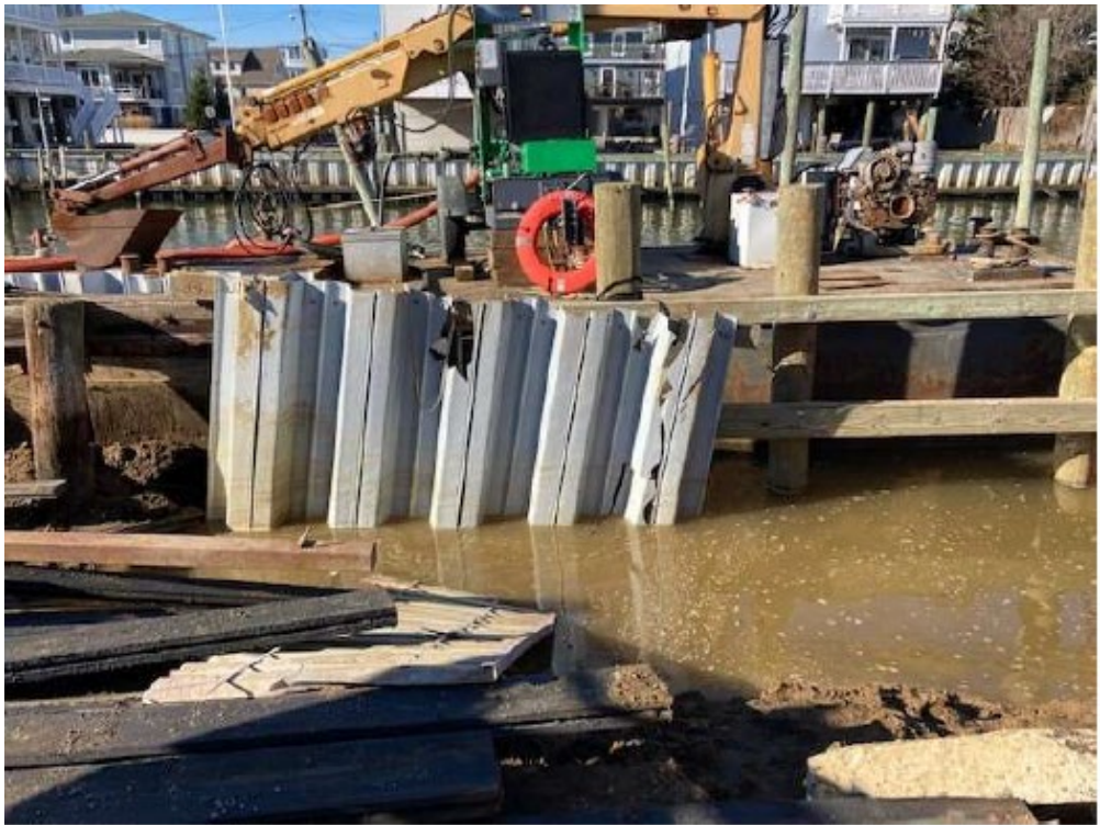
Road sub-base eroded into the cove (From Colliers Engineering and Design's Letter dated January 9, 2023)
