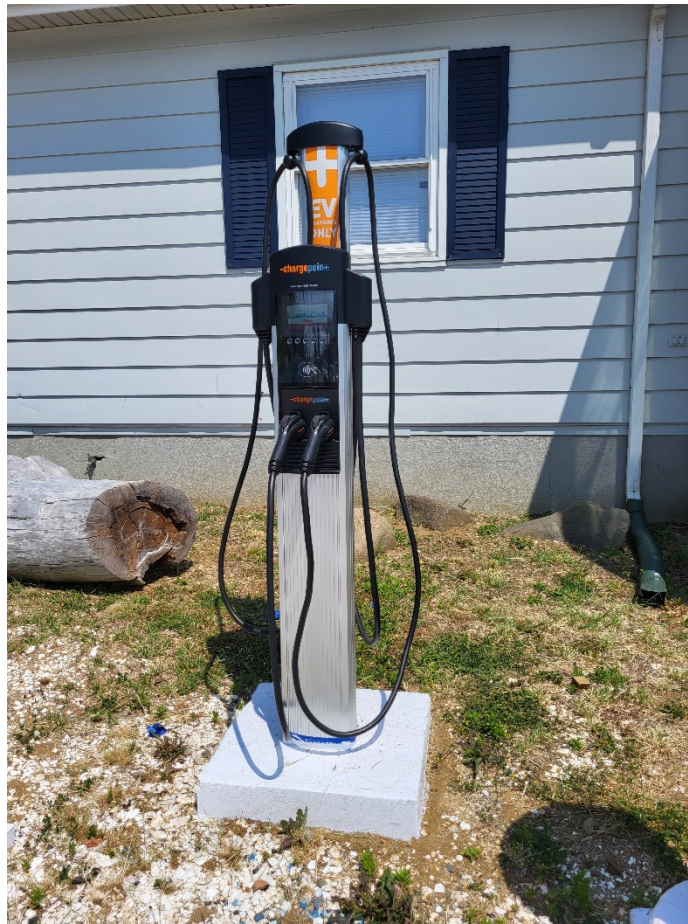
Photo 2: Existing EV infrastructure
