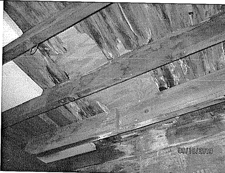
Photo No.: 8 (looking upward) Description: View of underside of second floor joists and flooring as seen from the first floor.
