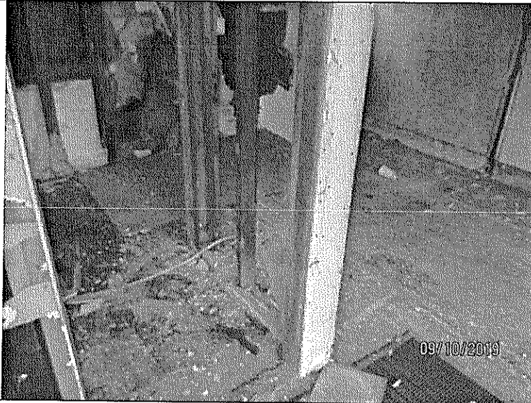
Photo No.: 5 (facing South) Description: General view of second floor timber flooring with plywood covering large opening in view.
