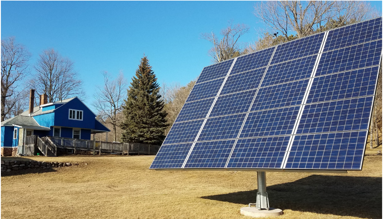
Ground-mounted monopole SES. Photo by Bradley Neumann.
