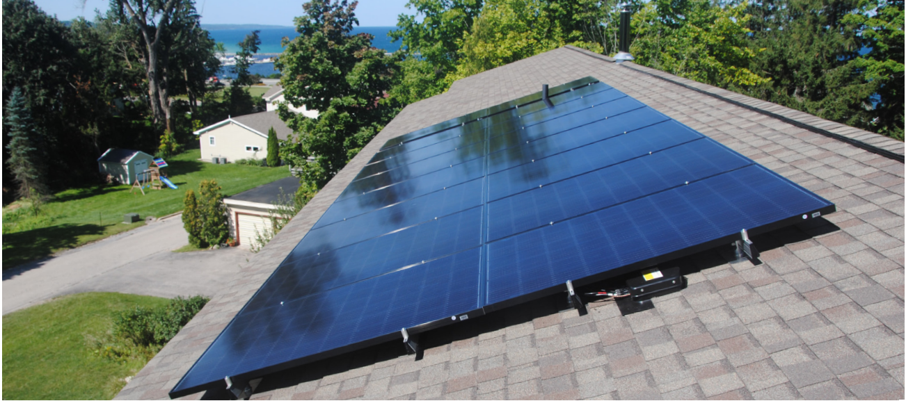
Rooftop SES, Petoskey, Michigan. Photo by Richard Neumann.
