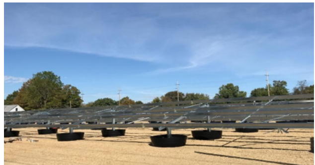
Coldwater Solar Field Park. Image courtesy of City of Coldwater, MI.
