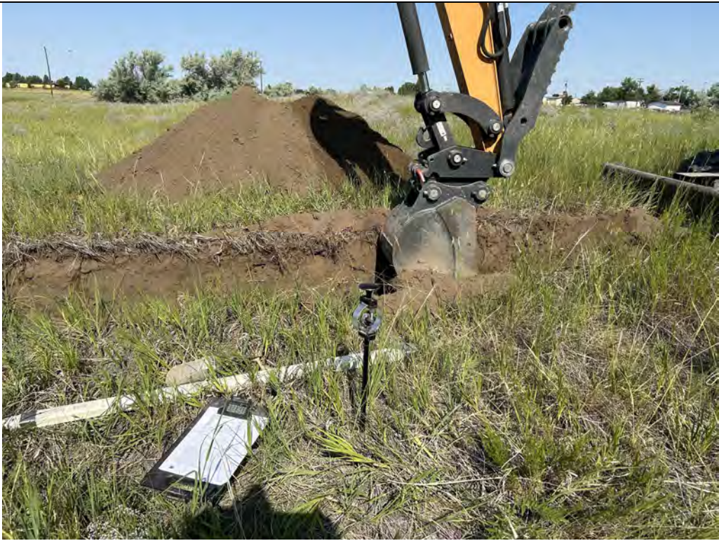
Description: TP-03 Location. Cone penetrometer was pushed 6 inches under a 320 psi loading.
