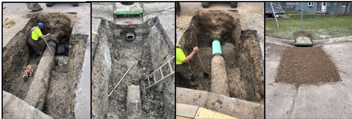
Routine inspections identified a damaged 12" inlet run; Utilities team repaired the inlet.
