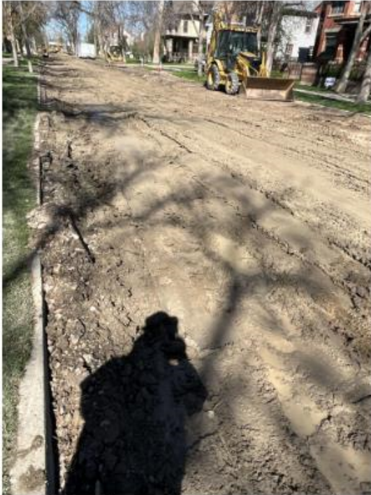
Rutted subgrade on 3rd Ave N. to be removed
