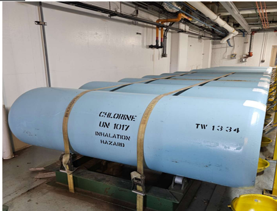
Figure 1: Chlorine Storage Room
