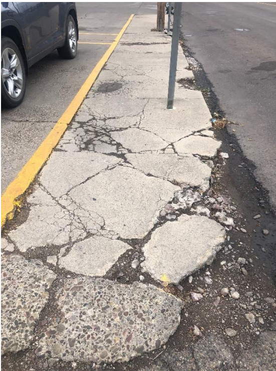
Broken sidewalk, missing curb
