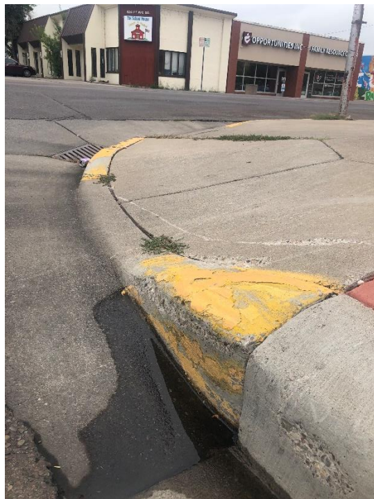
Non-compliant curb ramp
