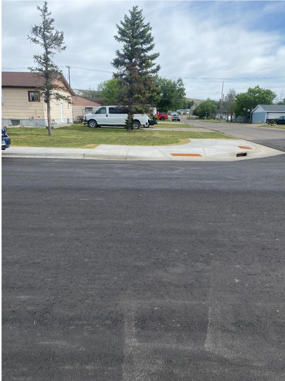
New sidewalk and road surface from Phase 1, 7th Ave NW at 12th St NW
