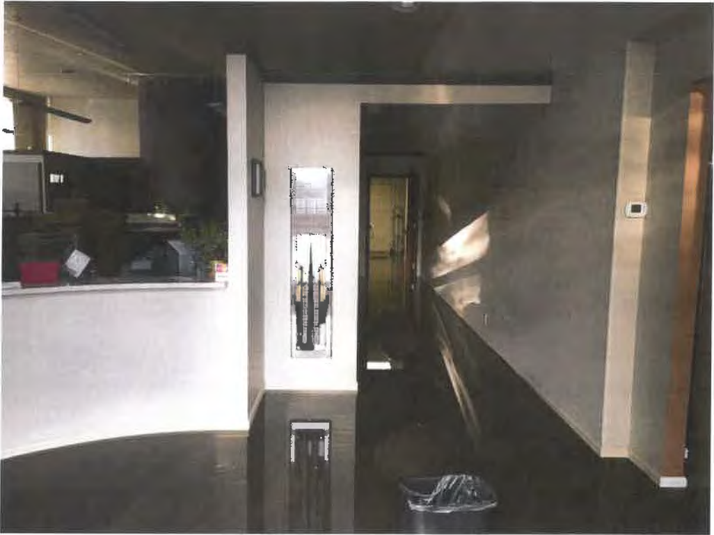
Flooding Inside Builders Exchange (8-9-16)
