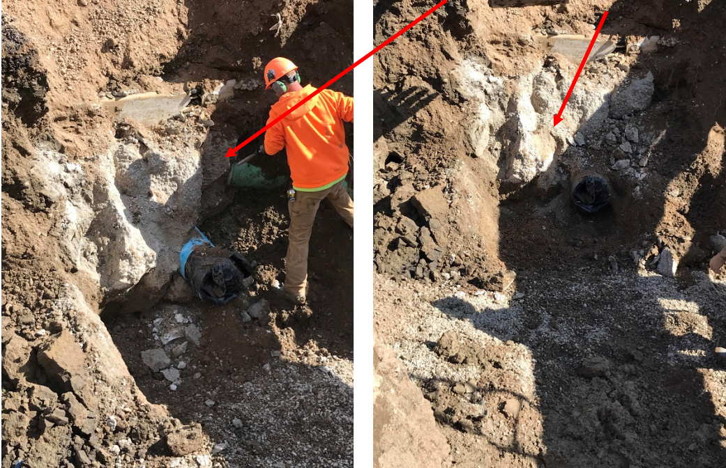
4+40 at the intersection of 3 rd St S and 3 rd Ave S inlet run encased in concrete
