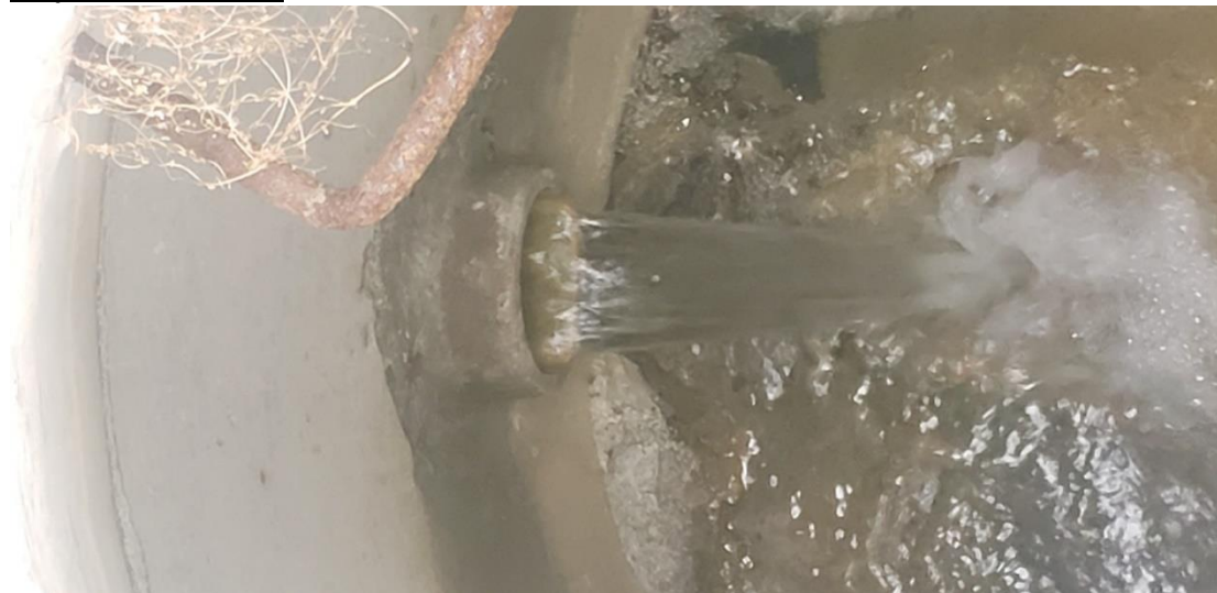
Figure 1 Foundation drain, approximately 50 gpm
