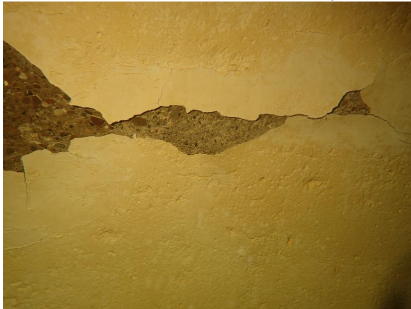
Figure 2 Cracks and flaking inside of tank
