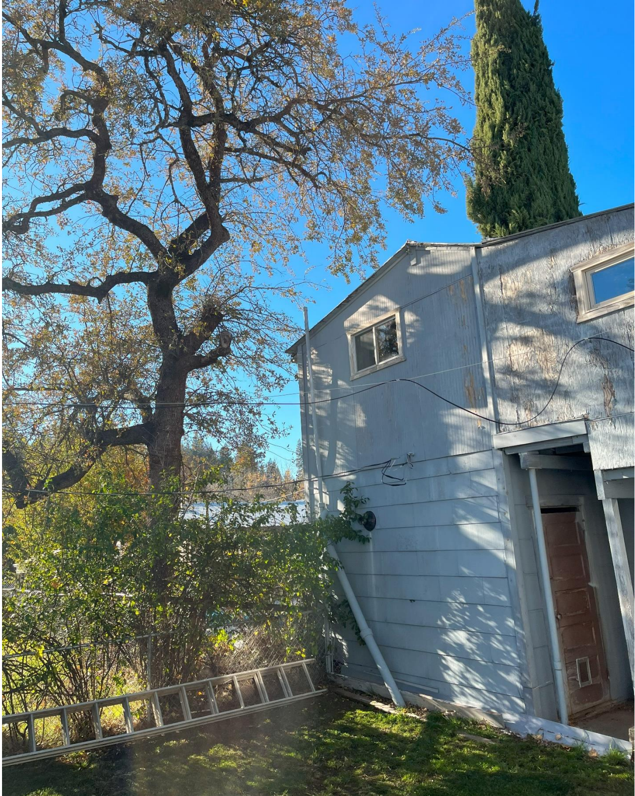
Photo 6: A two-story structure would require overhanging branches to be removed. The tree would be side heavy to the left and could fall or damage the foundation and/or the neighboring pool where the tree is rooted within the adjacent parcel to the Project.
