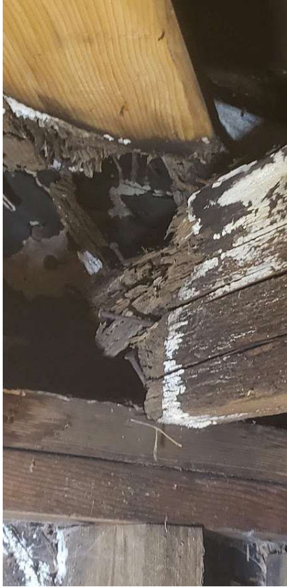
Figure 1- Deteriorated Floor Joist
