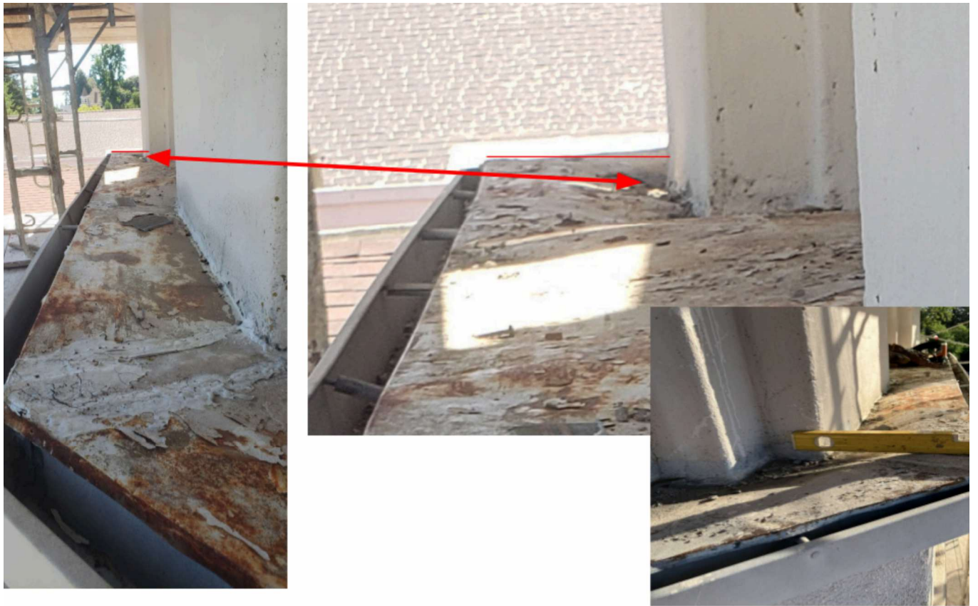
Figure 2- Greater than 1" settlement in the upper level of photo
