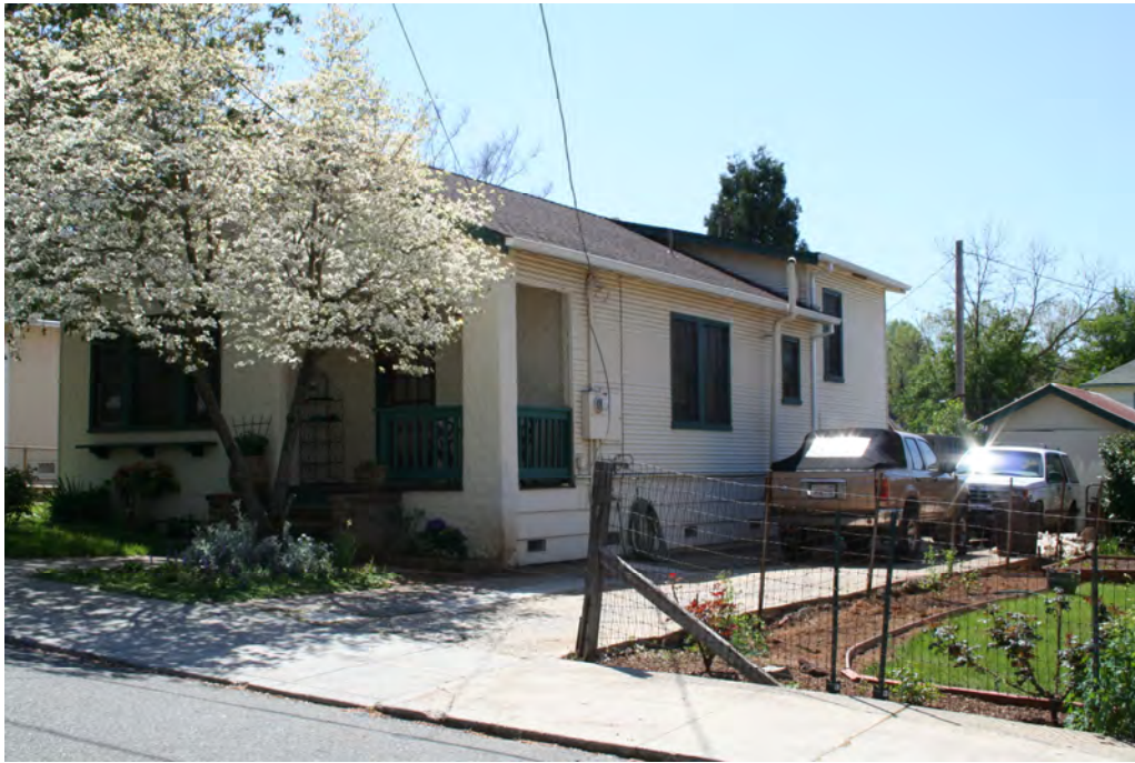
View looking southwest at the north elevation of the house. Note the rear shed roof addition.
