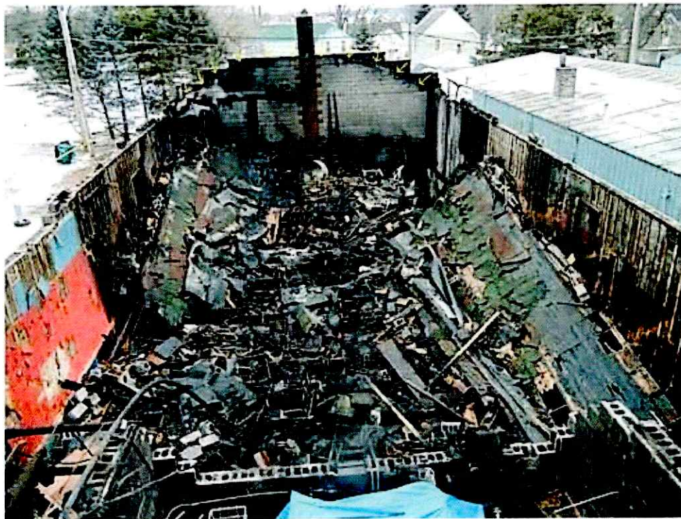
The catastrophic collapse of a truss roof during a fire
