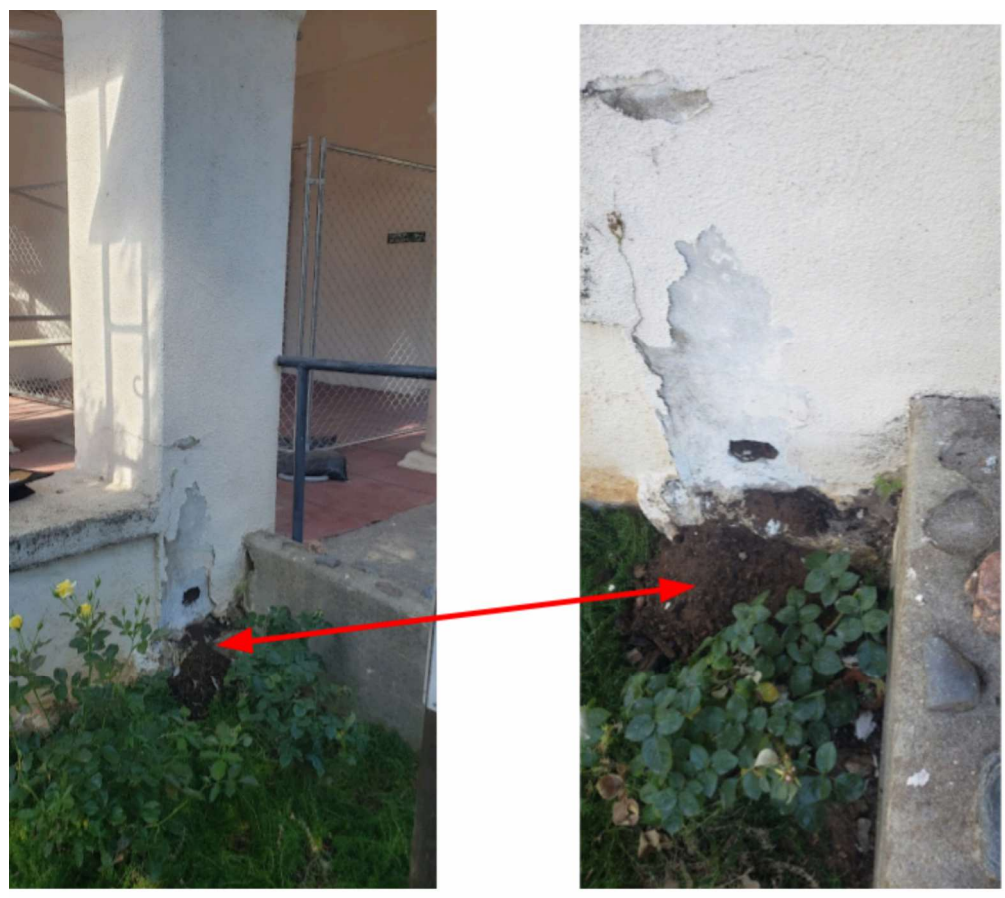
Figure 3- Wood debris from inside the easternmost column
