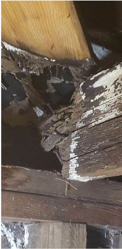
Figure 1- Deteriorated Floor Joist
