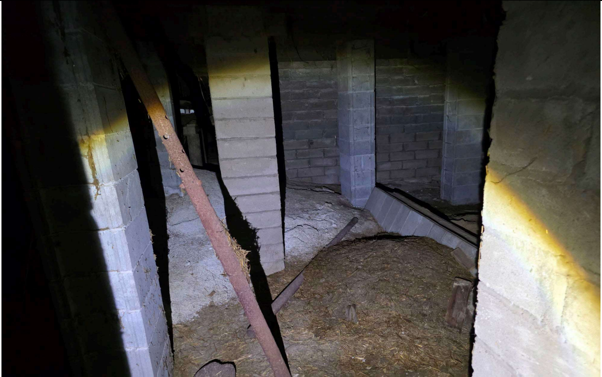
Photograph 37 Date: April 14 th , 2026 Direction: East Subject: Dirt floor area with an estimated 20-tons of unidentified fertilizer in the southwest portion of the Site building's basement bulk storage area.
