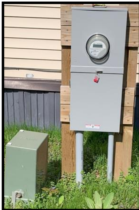
Figure 1: Ped with Meter base.
