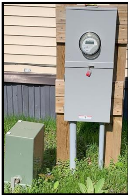
Figure 1: Ped with Meter base.
