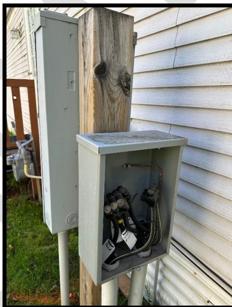
Figure 2: Junction Box with Meter Base
