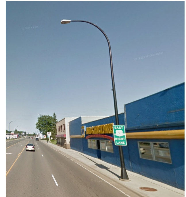
Standard Corridor Lighting in the Sidewalk
