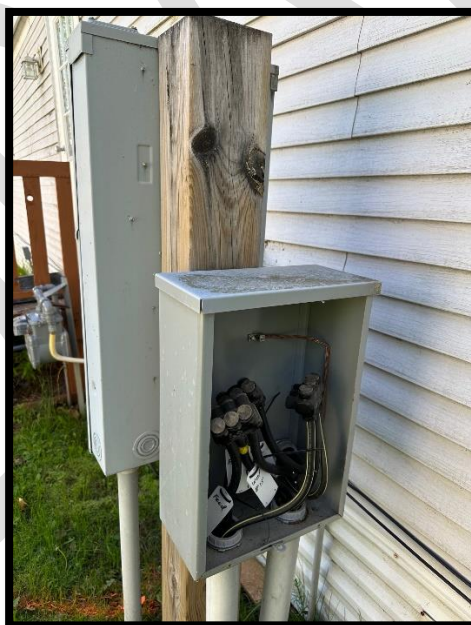
Figure 2: Junction Box with Meter Base
