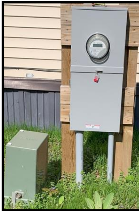
Figure 1: Ped with Meter base.
