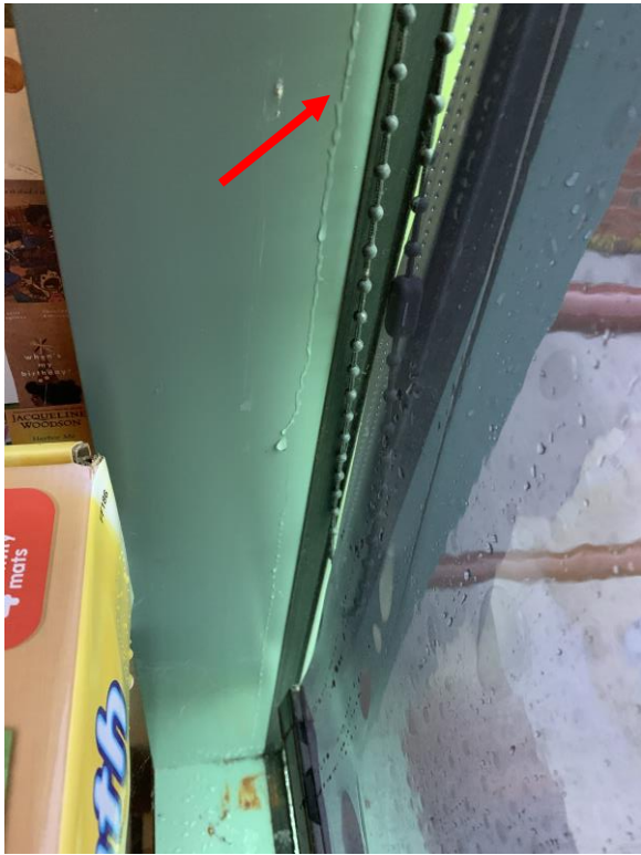
Photograph 8 – Leak location at the office window.
