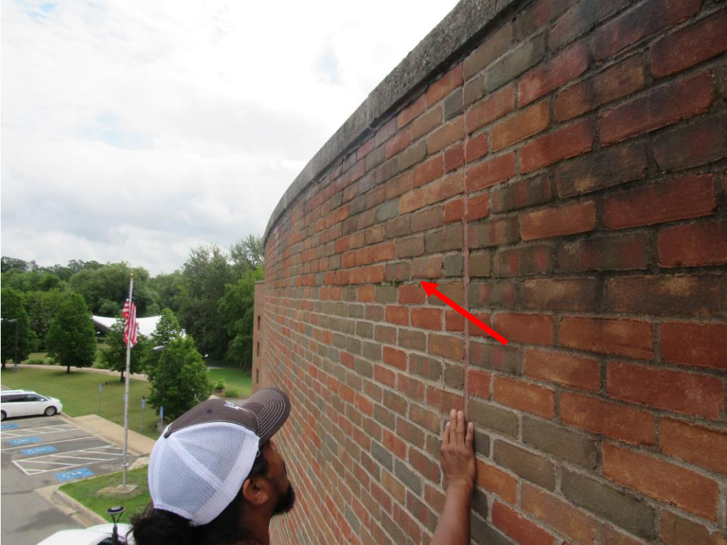
Photograph 14 – Water-stained masonry with cracking at bed joint. Moss formation is also noted.
