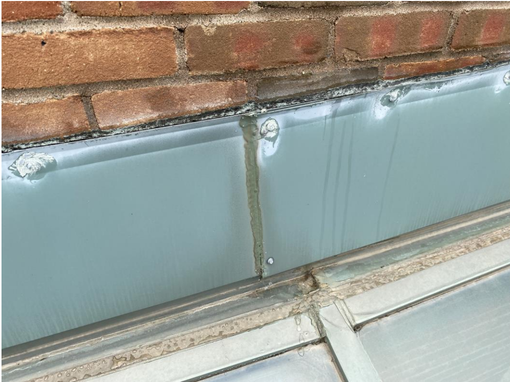
Photograph 21 – Failed sealant joints at the skylight wall flashing, no through wall detail is visible with existing wall flashing.
