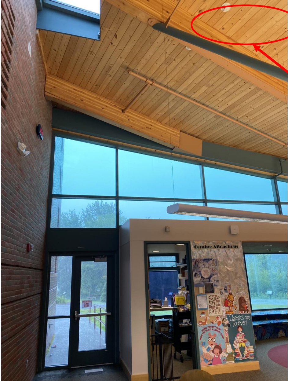
Photograph 9 – Reported leak location at the ceiling near the east entry doors.
