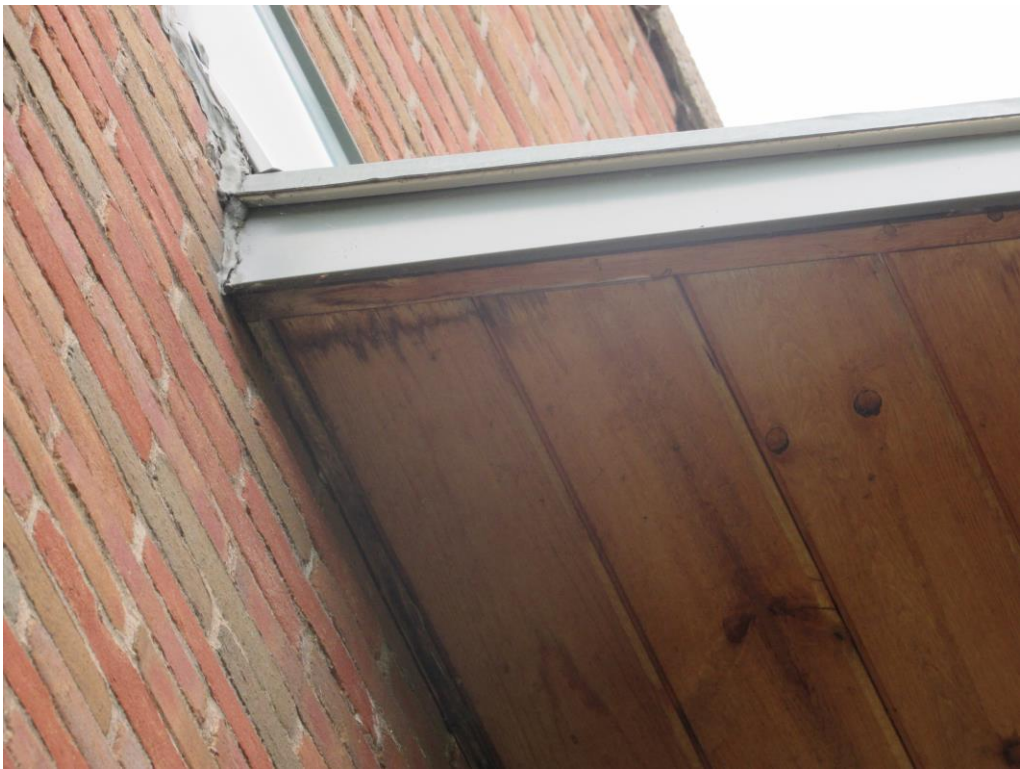
Photograph 17 – Water stains at a wood soffit.
