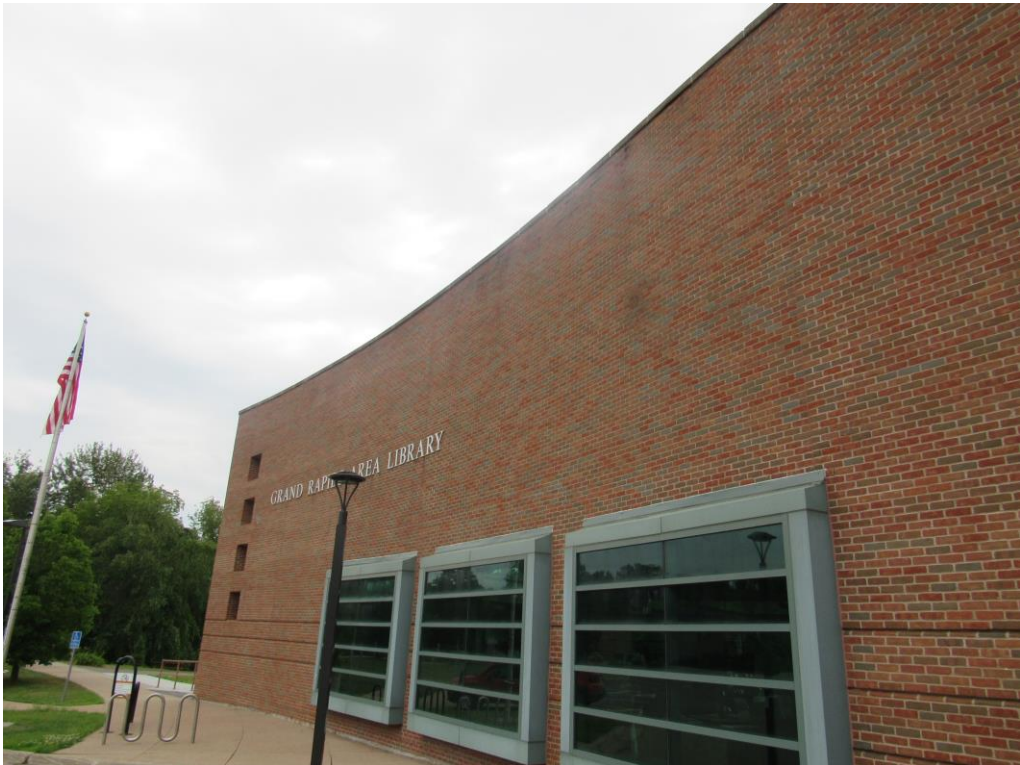
Photograph 11 – Typical masonry conditions at the north elevation.
