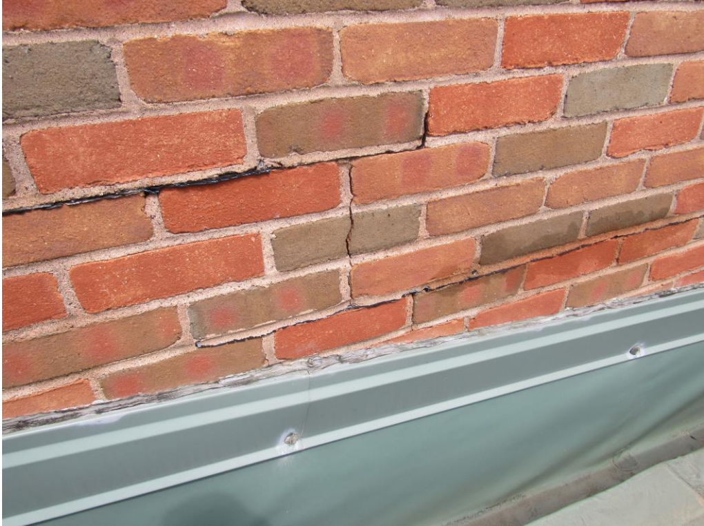
Photograph 16 – Brick crack around through wall flashing details.
