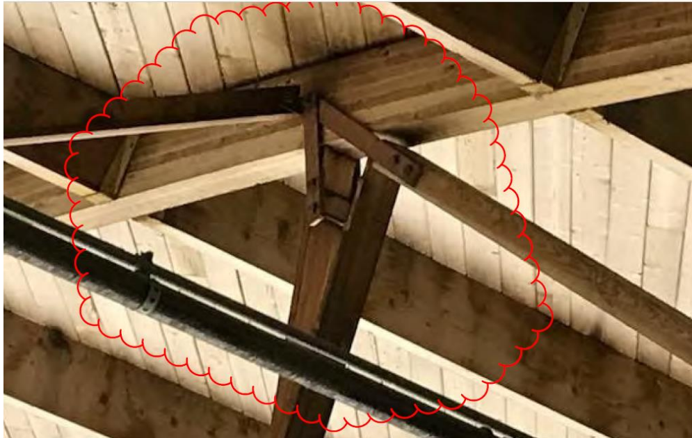
Picture of Failed Truss Member
