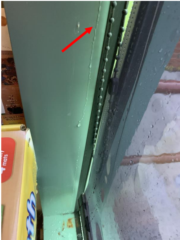
Photograph 8 – Leak location at the office window.
