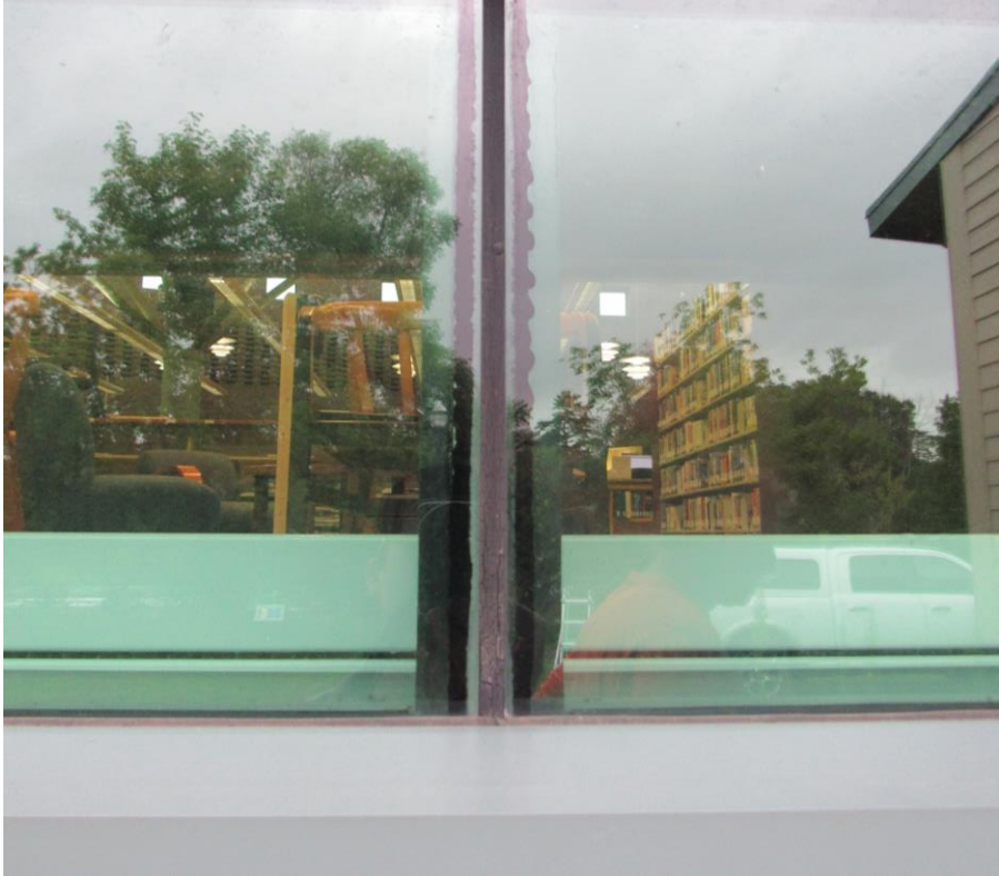
Photograph 18 – Cracking sealant at a window assembly.
