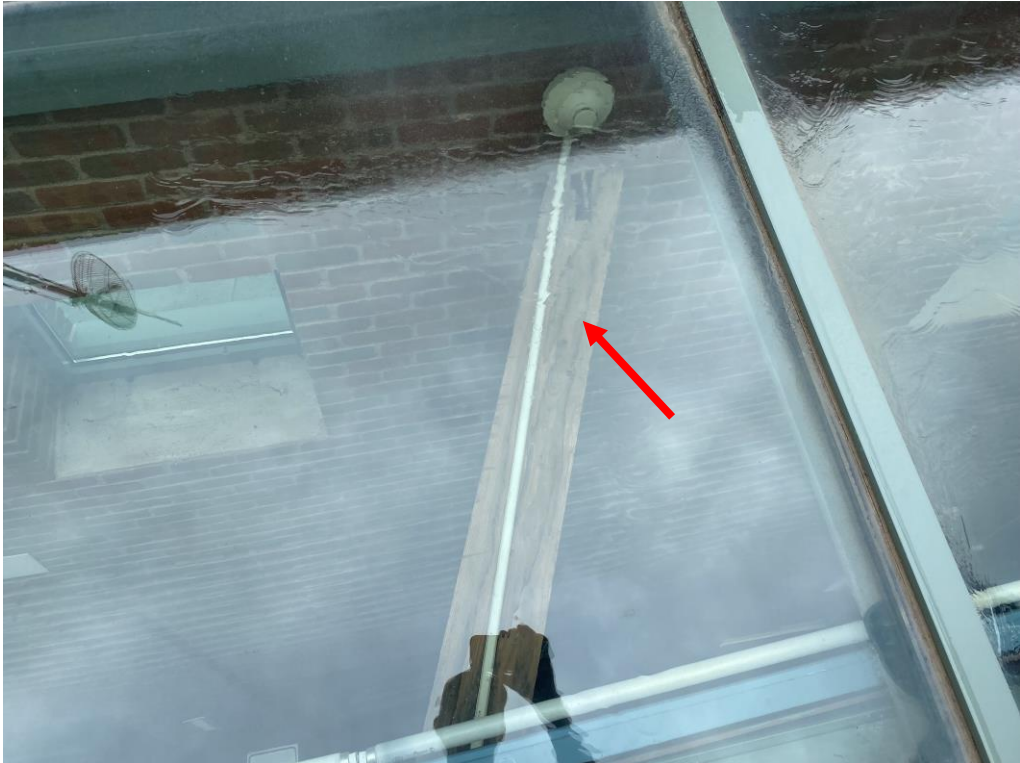
Photograph 23 – Water stains at the wood beam beneath the skylight.
