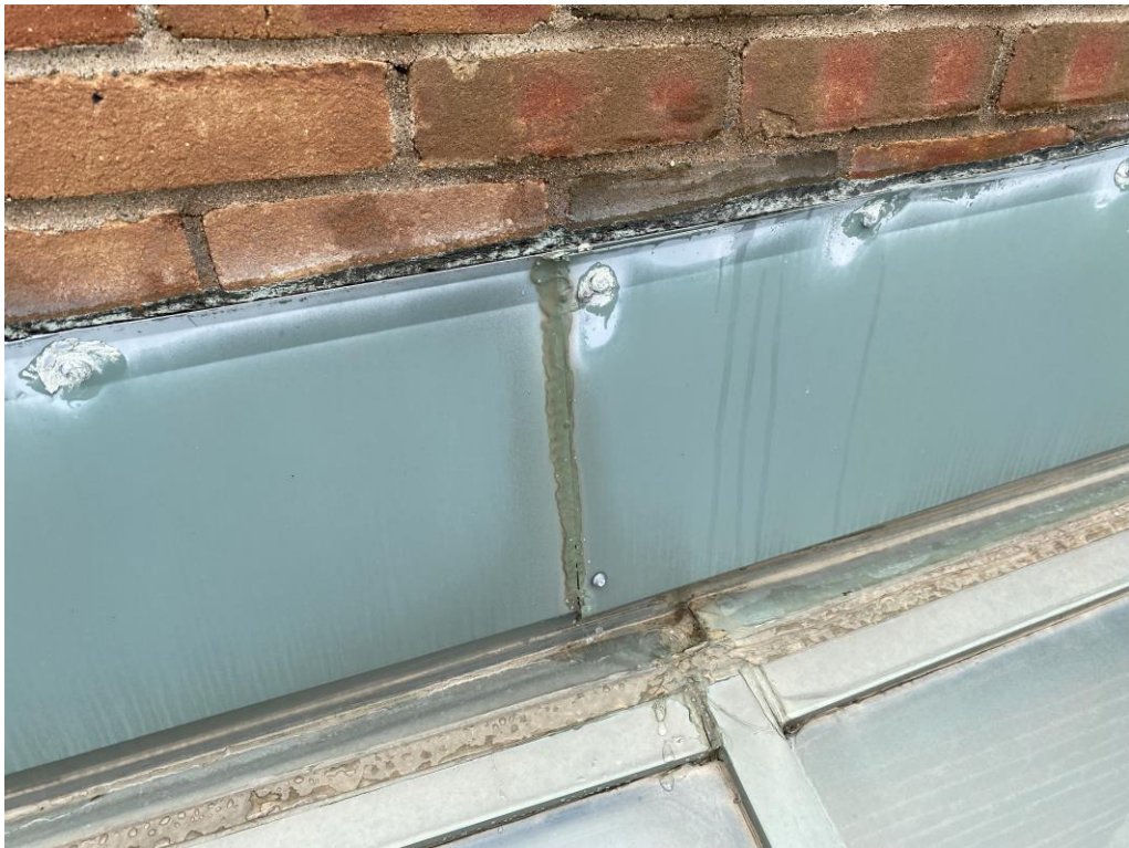
Photograph 21 – Failed sealant joints at the skylight wall flashing, no through wall detail is visible with existing wall flashing.
