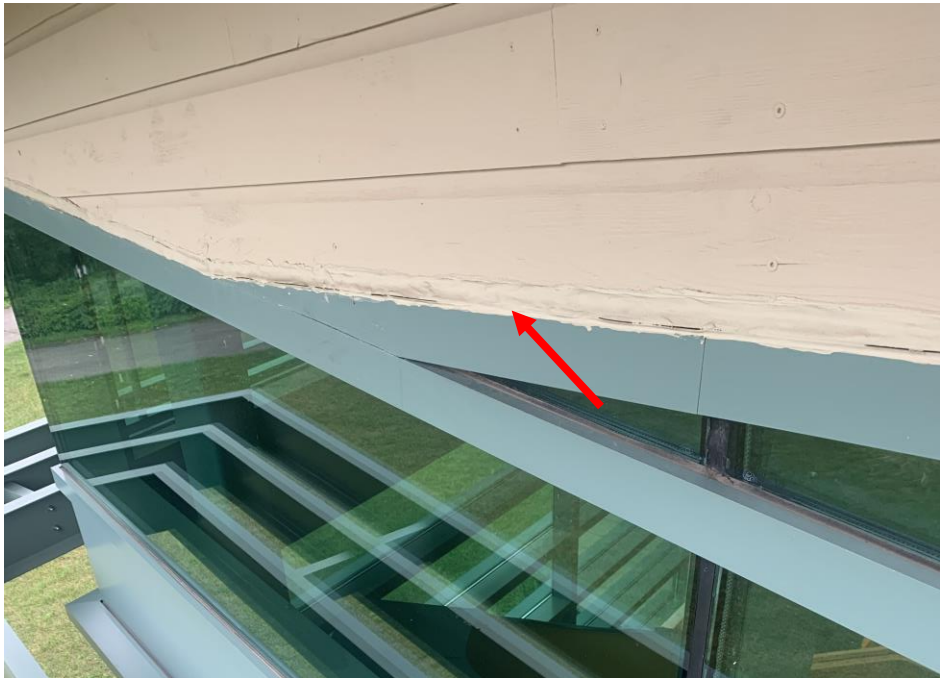
Photograph 25 – Sealant installed at window head/base of siding, with failures observed.
