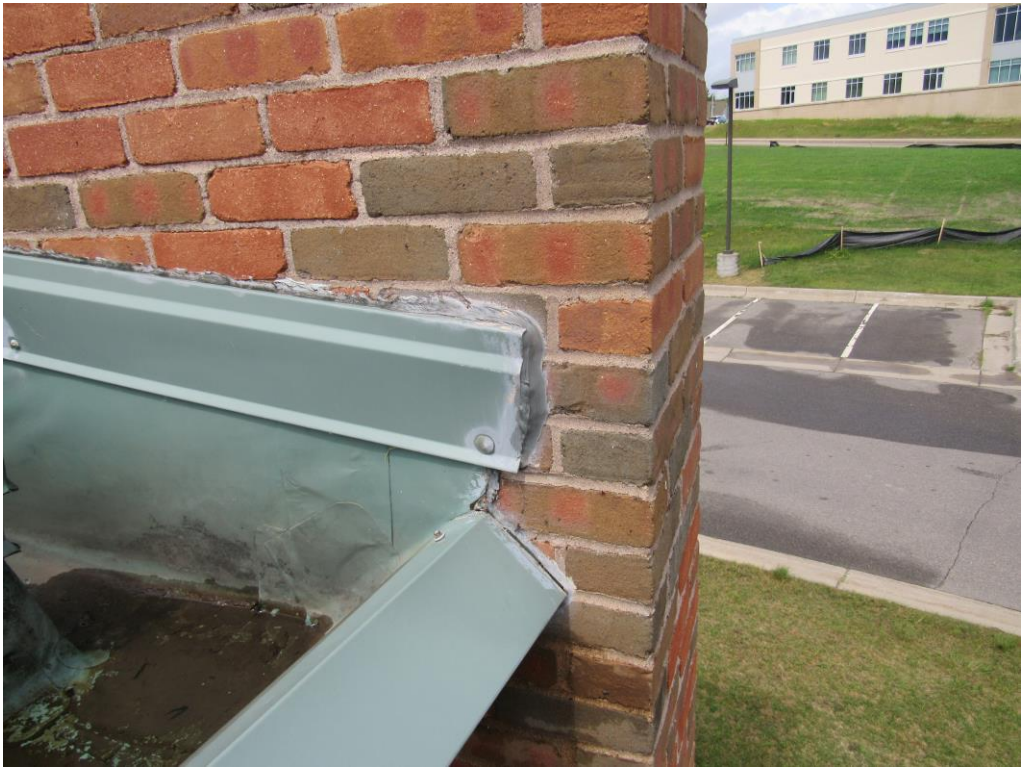
Photograph 27 – Failed sealants at metal flashings.
