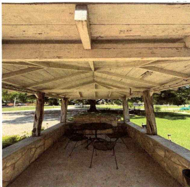
underside that will be repaired and replaced if need. Then painted from the approved color pallet.
