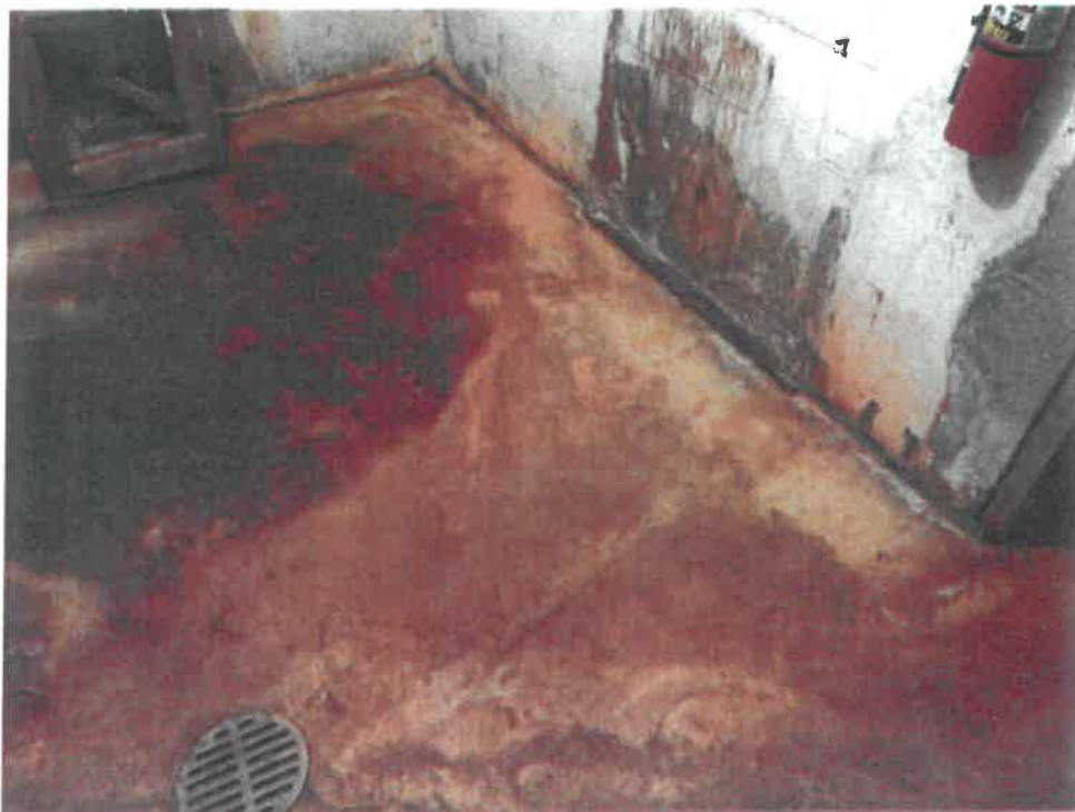
Photo 8: Perimeter French drains or baseboard drains and floor drain
