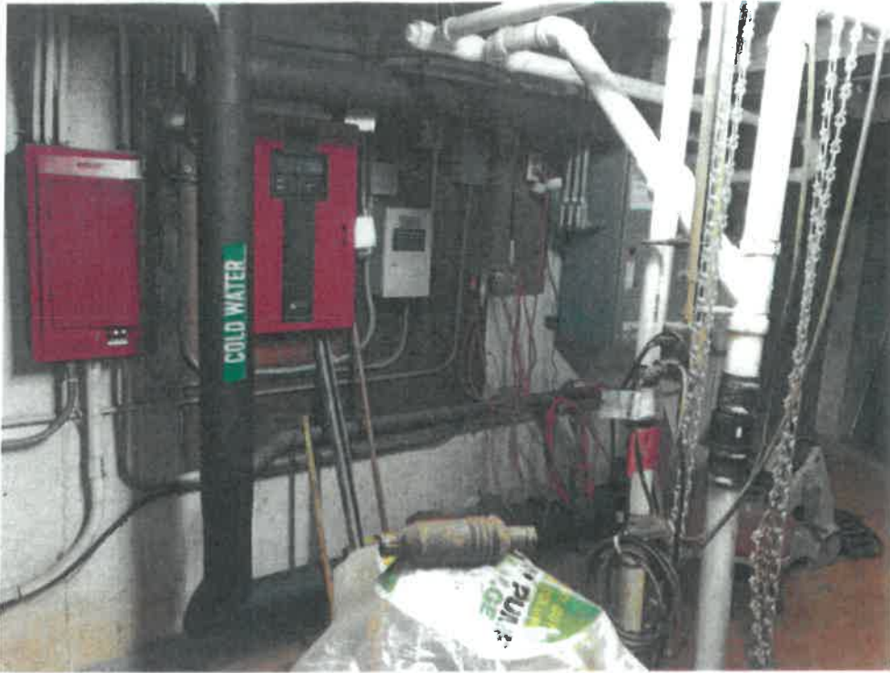
Photo 3: Electrical breaker boxes etc.
