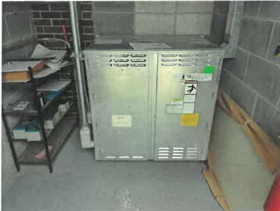
ELEVATOR OPERATING EQUIPMENT
