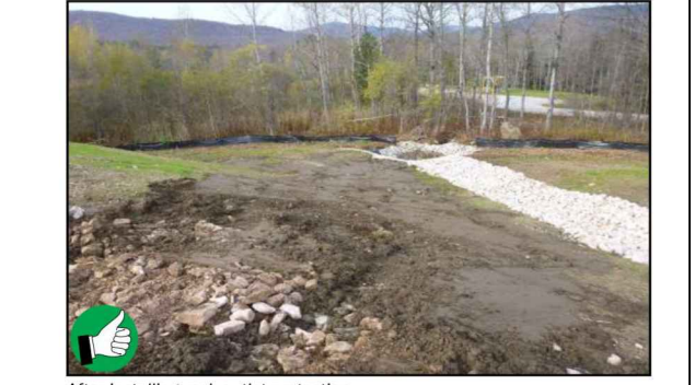
Stone riprap installed on an unstable slope with a stormwater outlet pipe along the slope. 45
