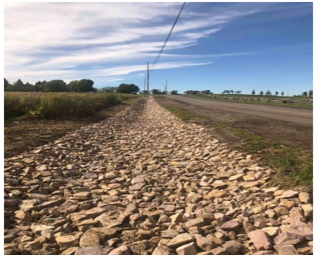
Figure 2.3: This new stone lined ditch on Kibbe Point Road was funded by Grants In Aid in 2022 and will reduce erosion and improve stormwater infiltration.
