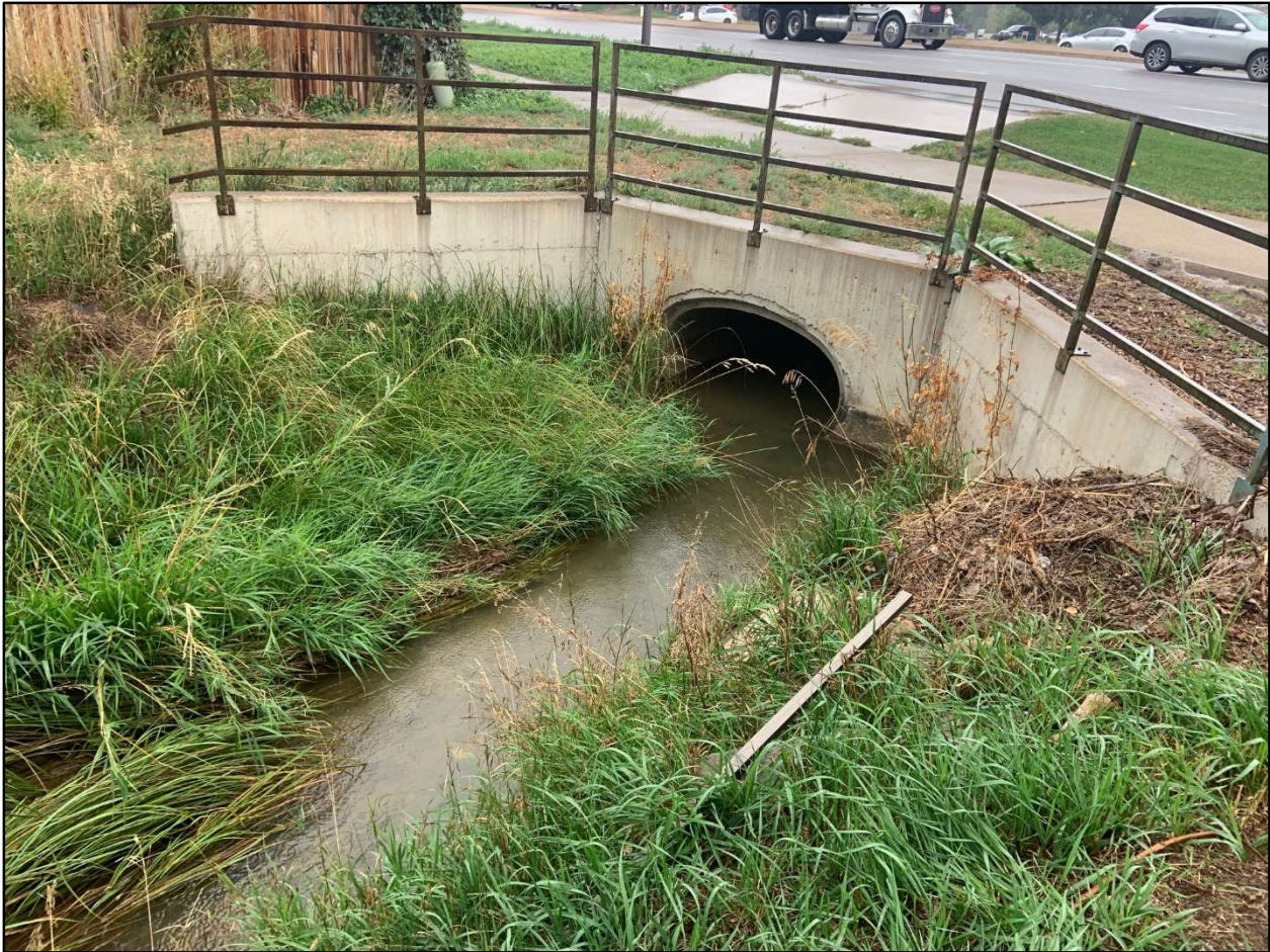
Photo 14. Timberline and Harmony: Dixon Canyon Lateral entering a culvert on the west side of Timberline Road at the intersection with Harmony Road. Banks were heavily vegetated with a mixture of upland and wetland vegetation.
