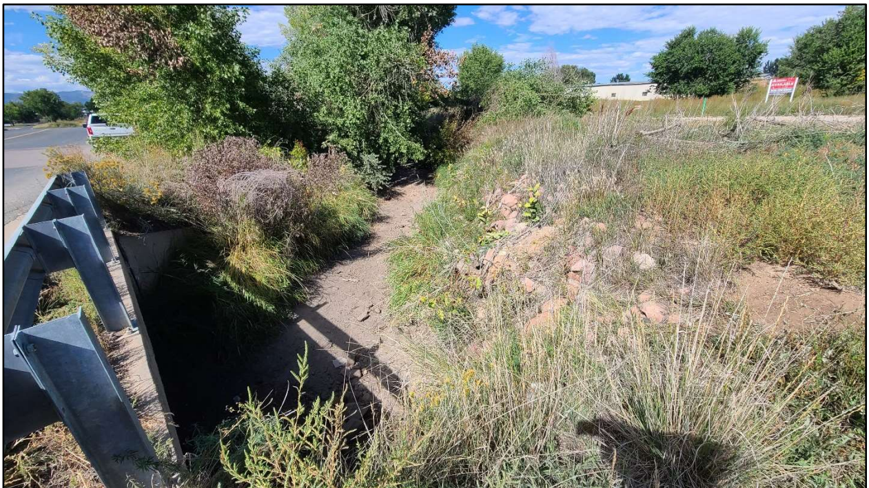
Photo 10. Timberline Road North – Segment 1: Northwest portion of Lake Canal on the Timberline Segment 1 project site. Canal was dry at the time of the investigation but still exhibited wetland vegetation.
