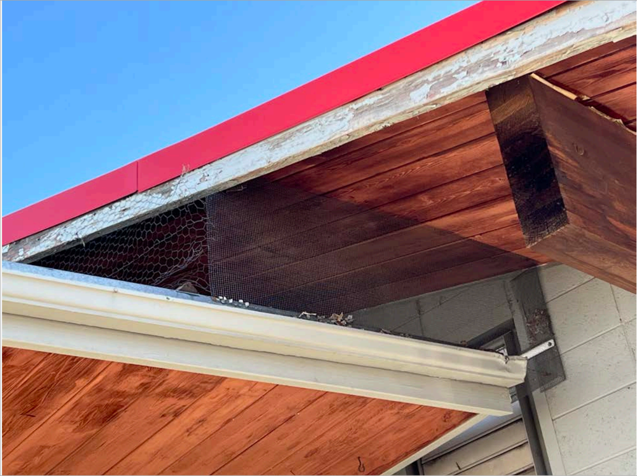
27. West Elevation - Back wall of the Showroom. Note netting at the eaves. Image courtesy of BEE. 2024.
