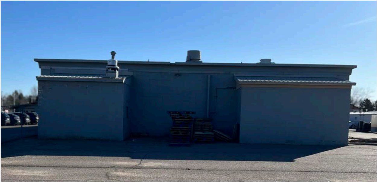
25. West Elevation - Back wall of the Service Center. Image courtesy of BEE. 2024.
