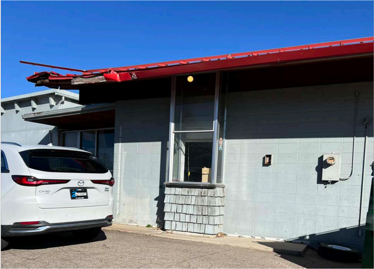
38. South Elevation - Showroom, "Bay window" that appears to have served as a drive-thru window. Image courtesy of BEE. 2024.
