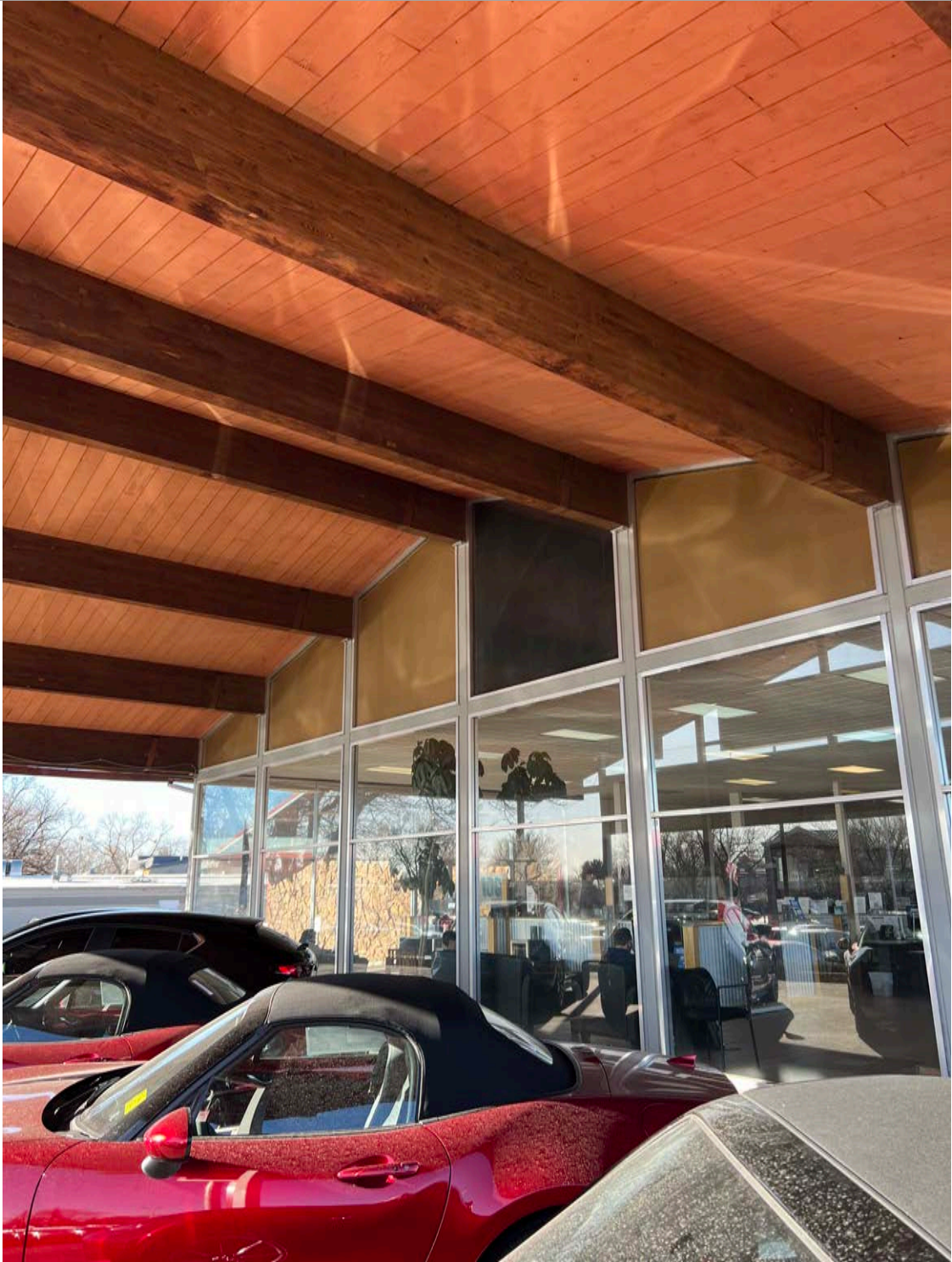
6. East Elevation - windows showing change in materials from installations of suspended drop ceiling on the interior. The original glass is missing, and the new material constitutes an intrusion. Image courtesy of BEE. 2024.
