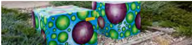
46 painted transformer cabinets
