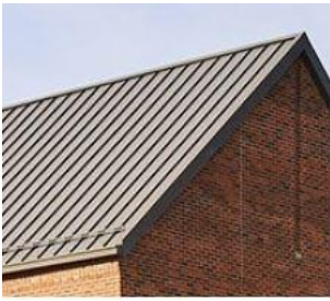
Roof: Gable Roof (Standing Seam Metal) & Flat Roof Brick and Stone (Cast Stone)
